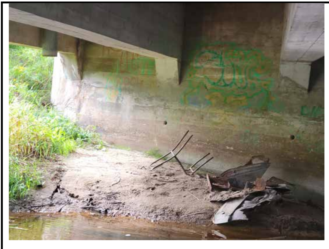
Photo 16 NW embankment encroaching into stream, accumulating debris
