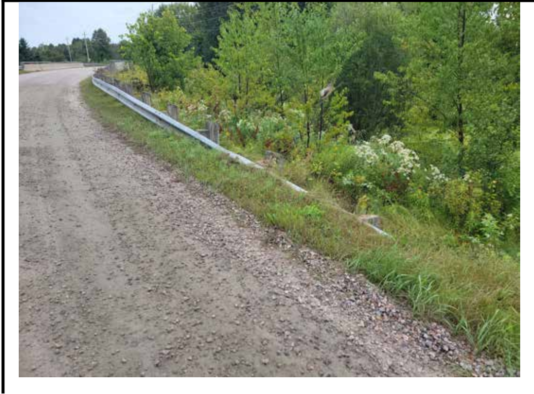
Photo 9 Substandard end treatment with weathered posts at SE corner of structure
