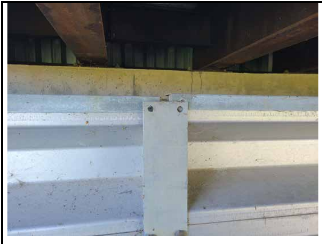
Photo 14 Missing bolts at south abutment wall
