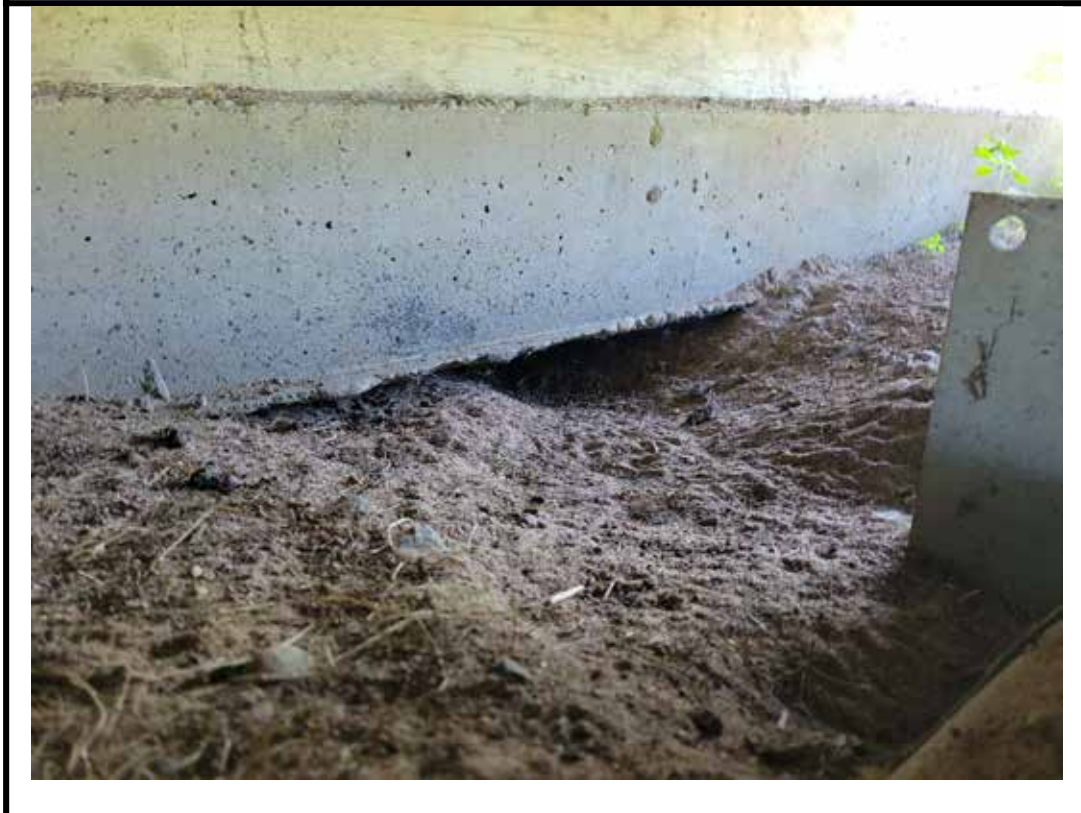
Photo 13 Undermining at concrete bearing seat cap at south abutment wall
