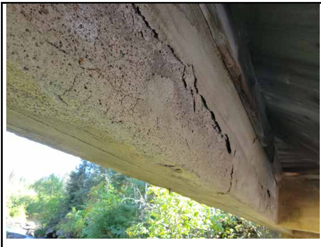
Photo 16 Light concrete disintegration on concrete girder
