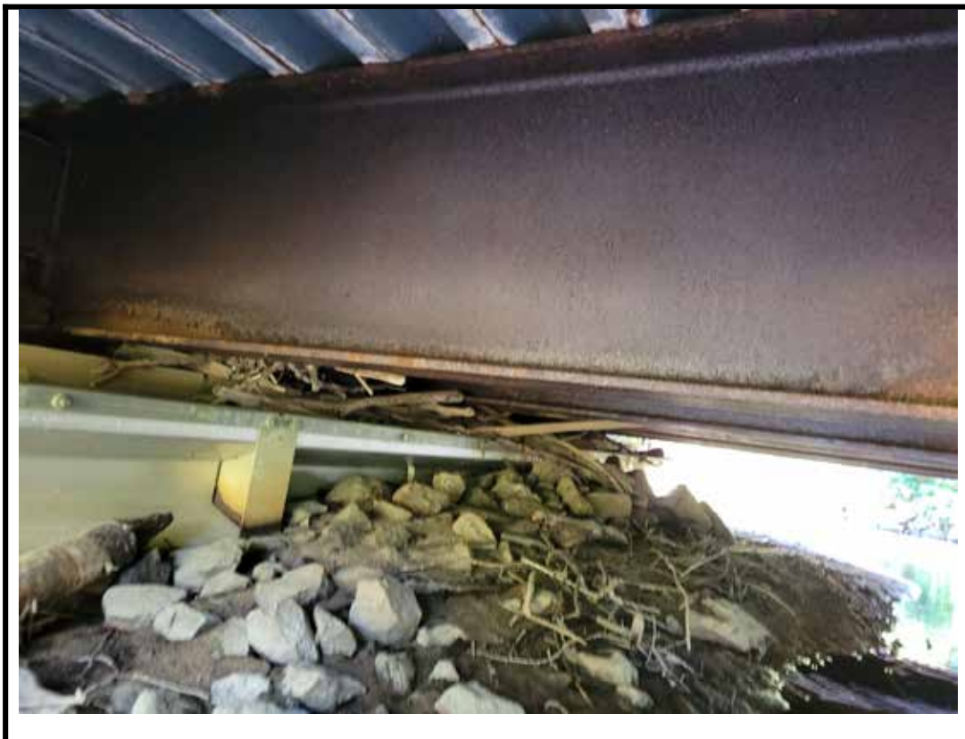
Photo 12 Accumulation of branches and debris at abutment
