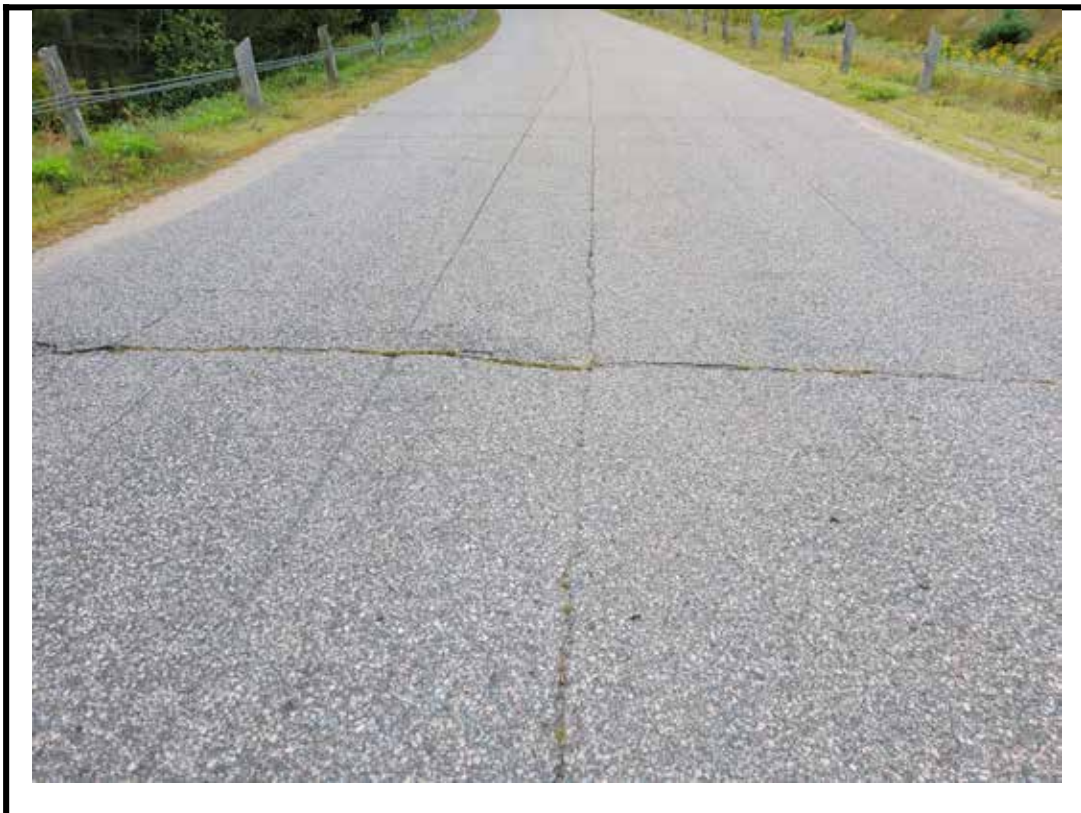
Photo 8 Longitudinal and transverse cracks on asphalt wearing surface
