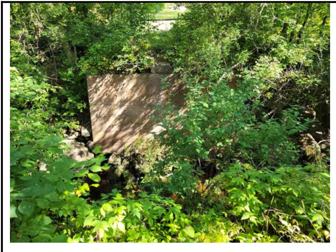
Photo 4 South abutment remaining
