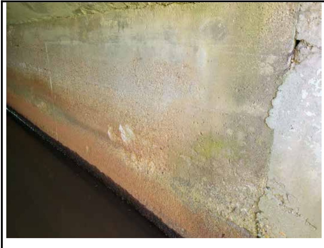
Photo 9 Localized honeycombing and small spalls at north end repair construction joint
