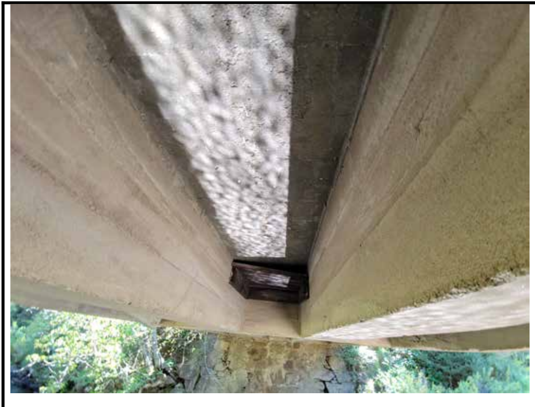
Photo 14 Light to moderate scaling on exposed deck soffit
