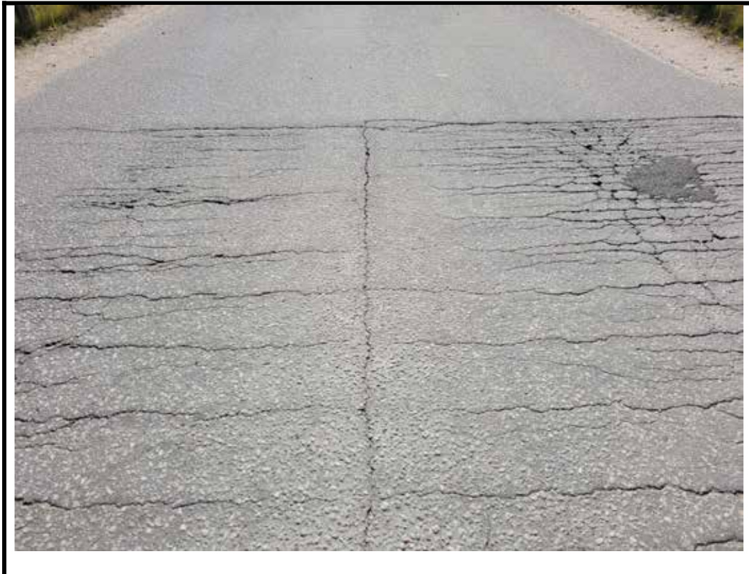
Photo 9 Wide cracks and patched pothole on deck top
