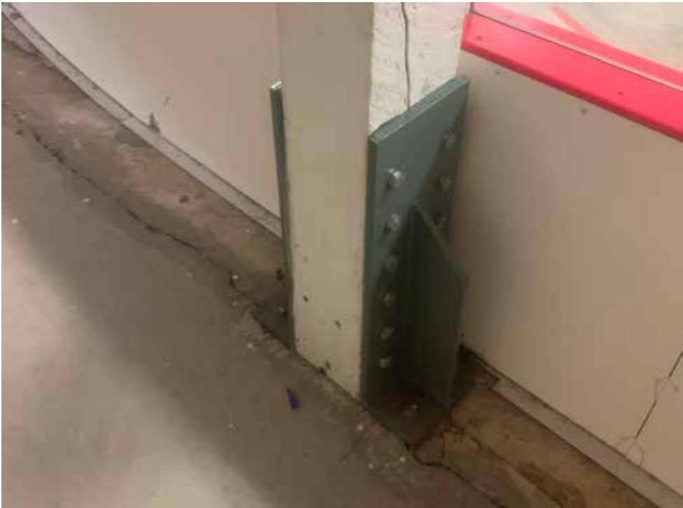
Photograph 3: Retrofit bolted steel plates - interior column
