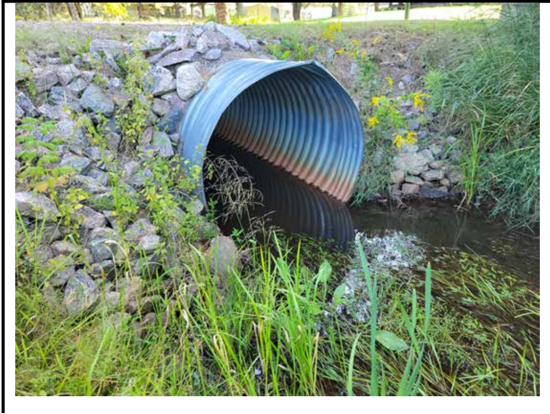
Photo 7 Deformation at north end of barrel
