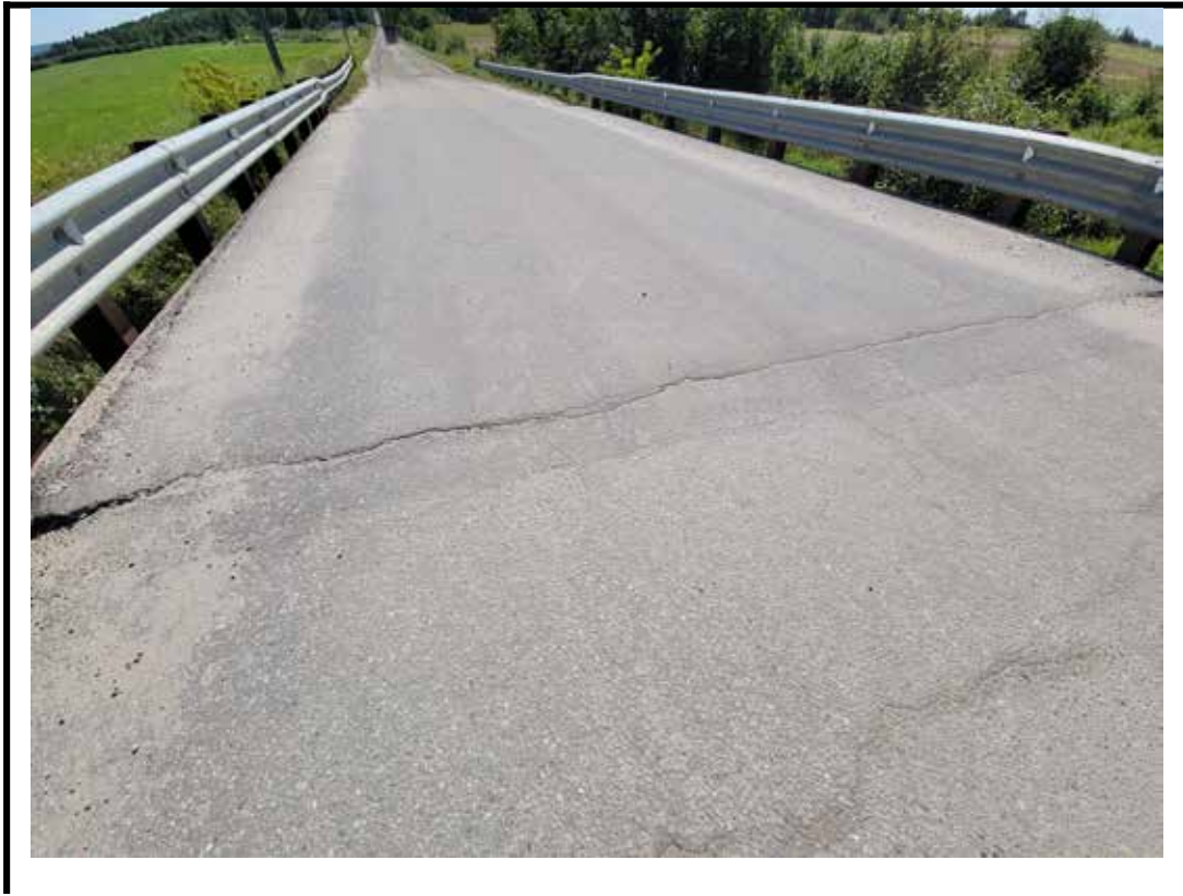
Photo 9 Transverse cracks noted on approach wearing surface at transition to deck
