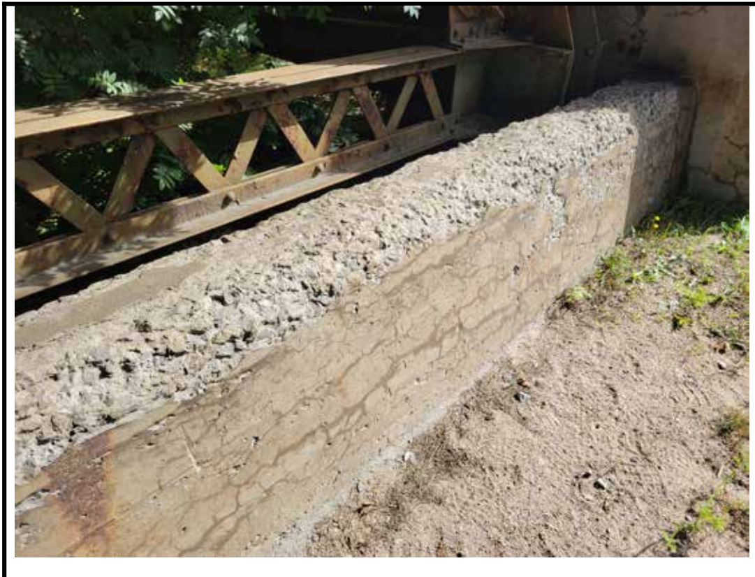
Photo 4 Light to moderate deteriorated on top of concrete crash wall
