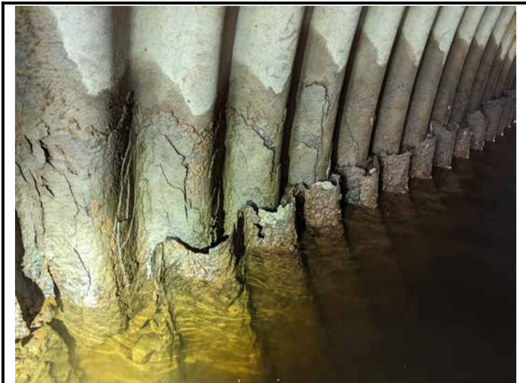
Photo 10 Severe corrosion with perforation and detachment on culvert barrel
