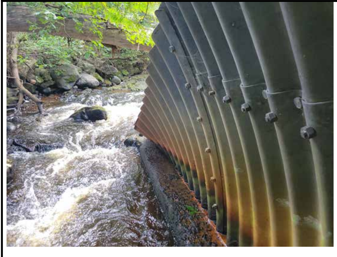
Photo 13 Deformation of east end of barrel
