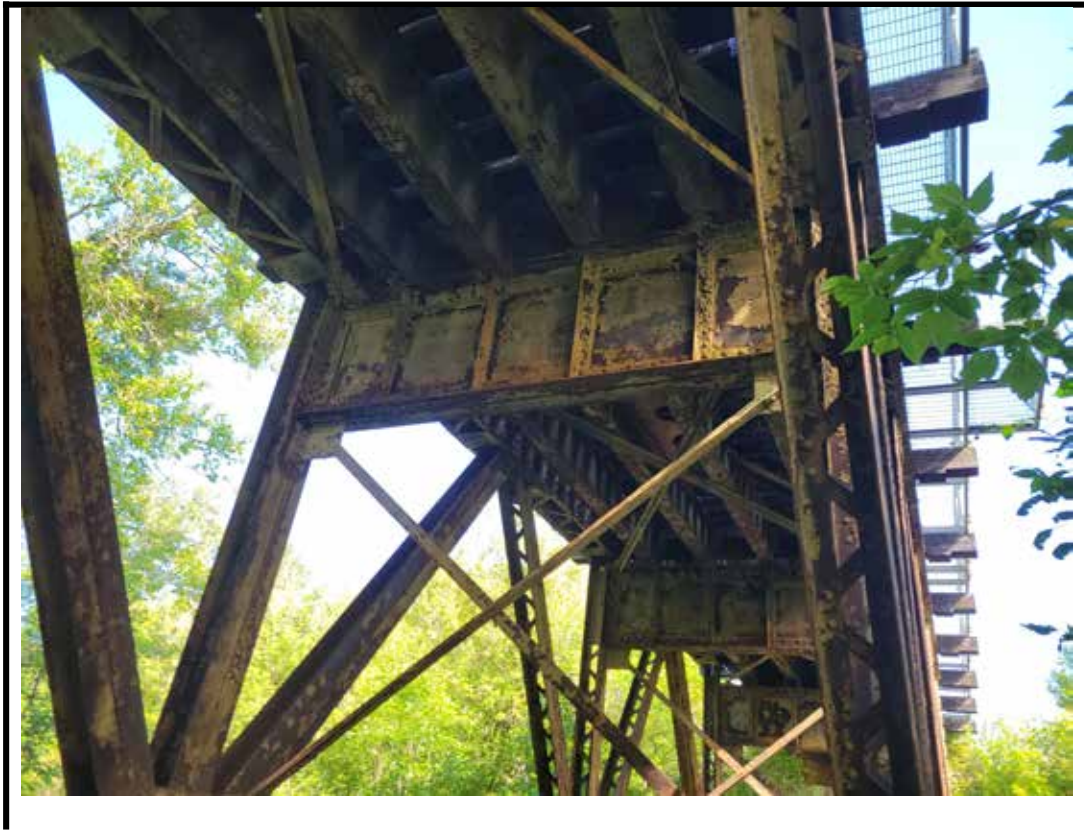
Photo 9 Coating failure and light to moderate corrosion on center span structural steel
