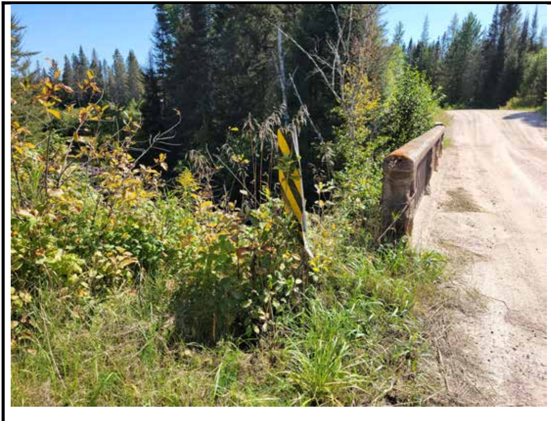
Photo 8 No approach barrier present at NE corner of structure & leaning hazard sign
