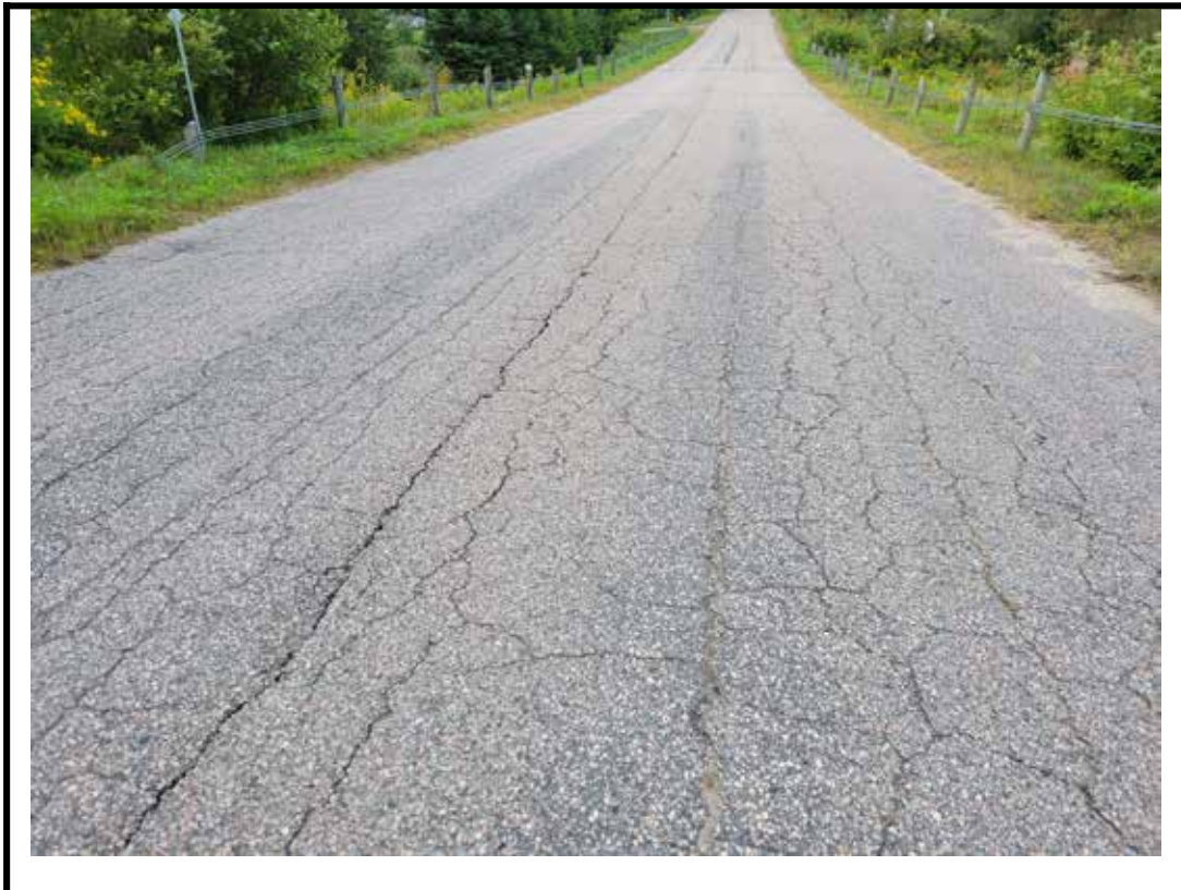
Photo 8 Longitudinal and transverse cracking on north approach wearing surface
