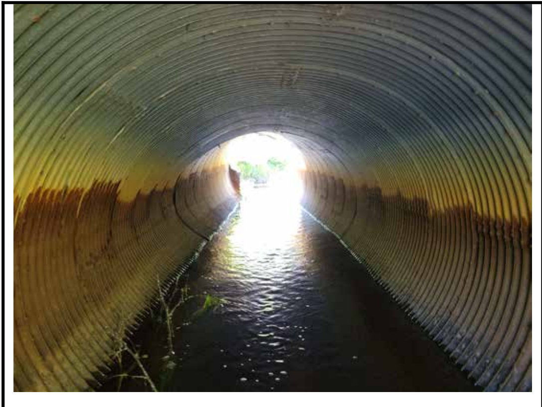
Photo 8 Sag at mid span of culvert barrel
