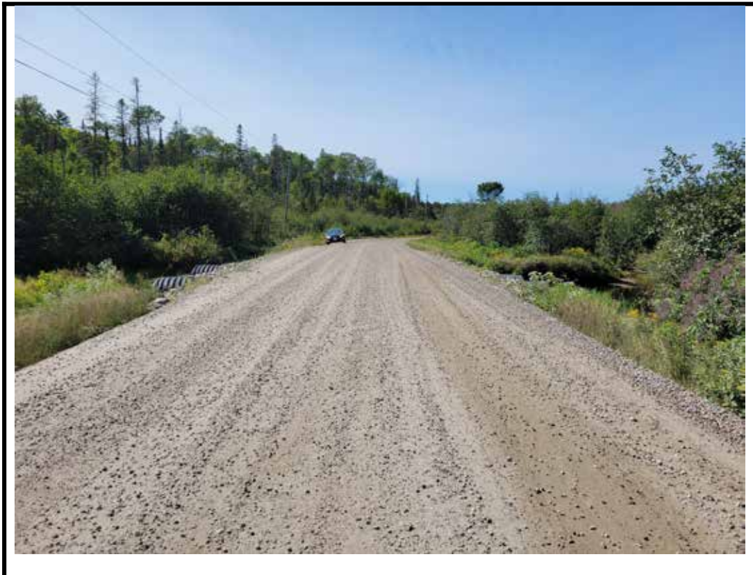
Photo 2 Structure from west approach
