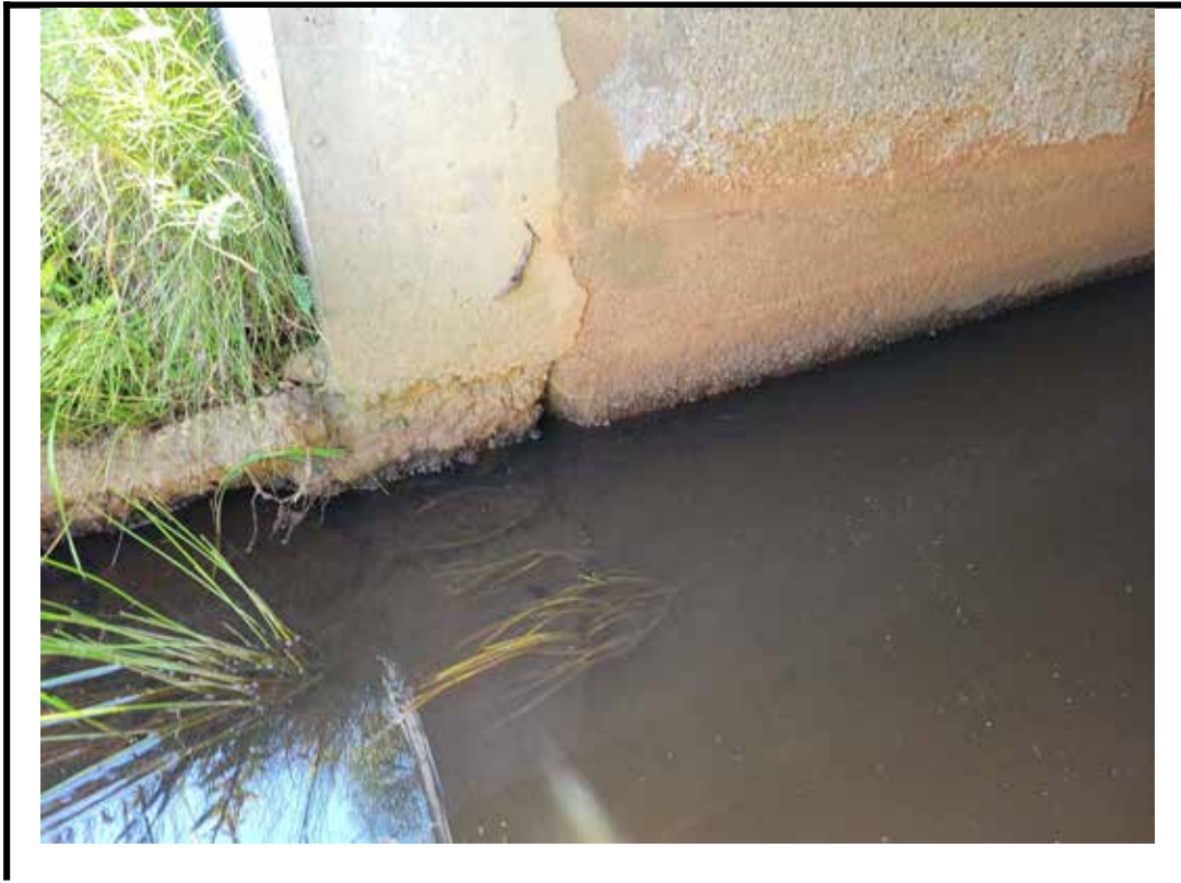
Photo 11 Localized light disintegration at base of reconstruction at SW corner of barrel
