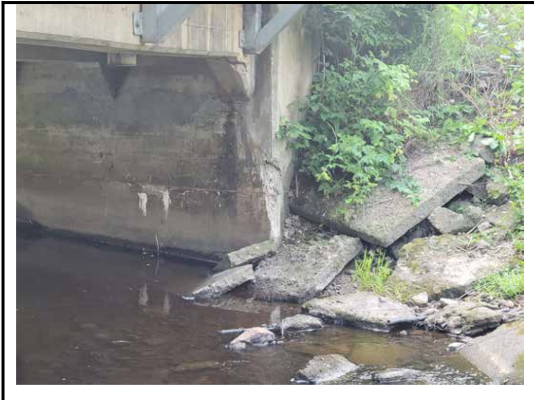
Photo 12 Localized severe deterioration of NE wing wall
