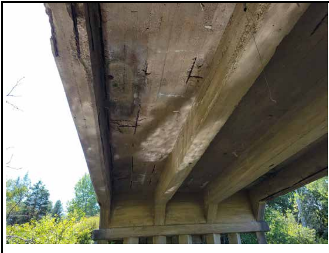
Photo 12 Severe spalls with exposed corroded reinforcing on mid-span girders and soffit
