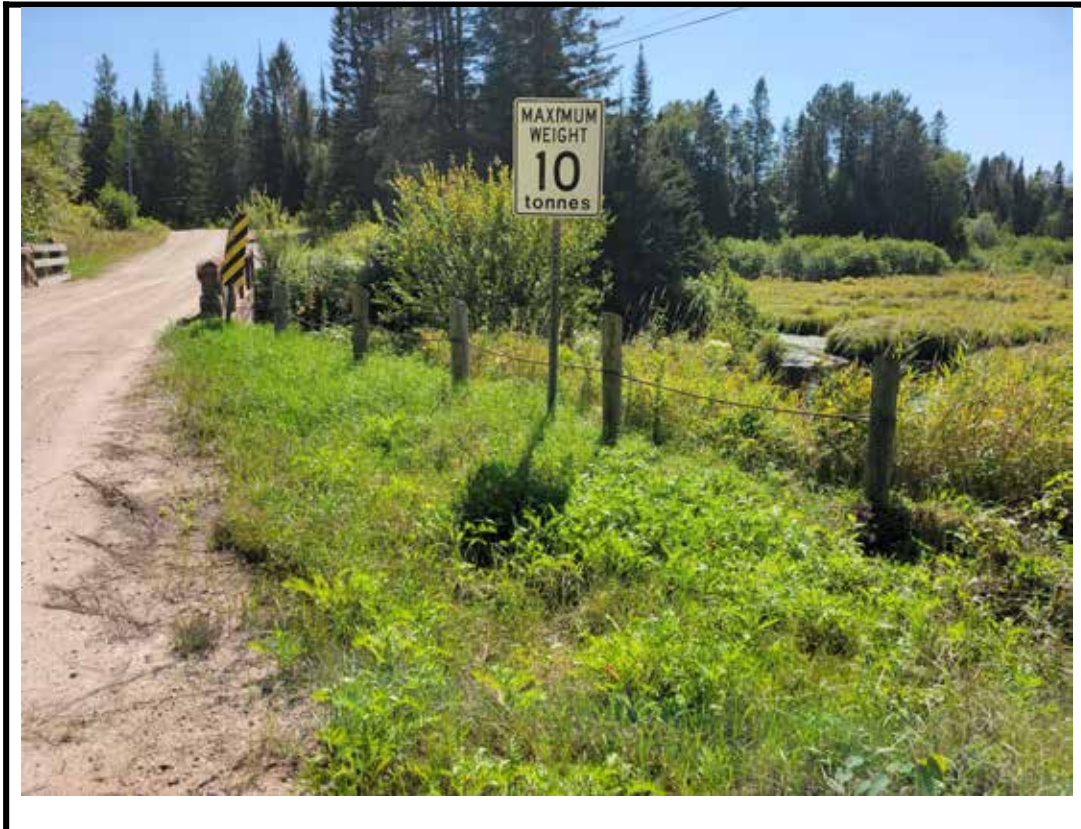
Photo 7 Substandard single cable guiderail on NW approach
