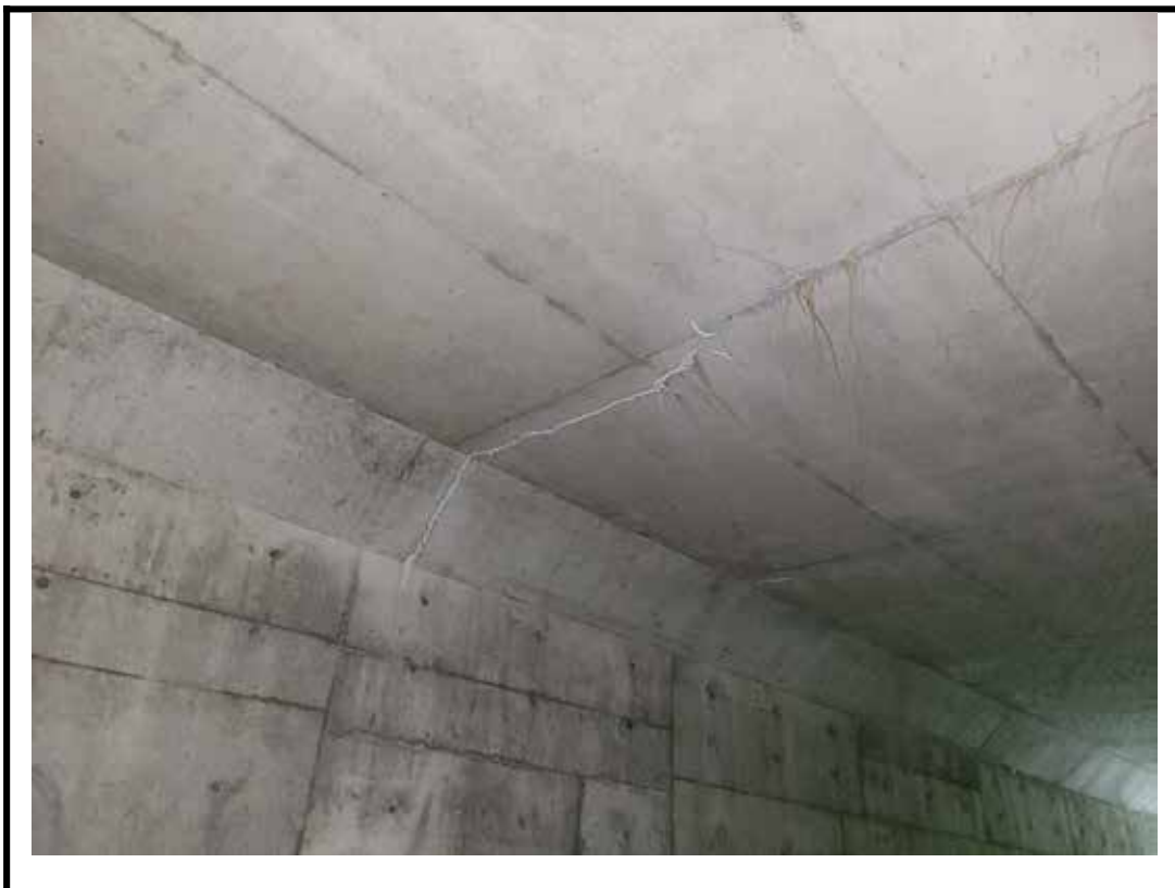
Photo 14 Narrow crack with efflorescence on soffit, west end of barrel
