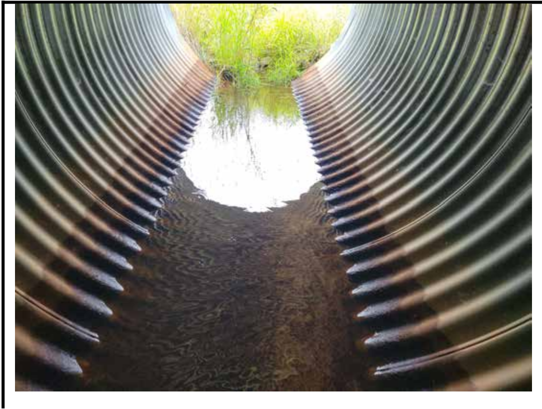
Photo 9 Light corrosion on culvert barrel at waterline
