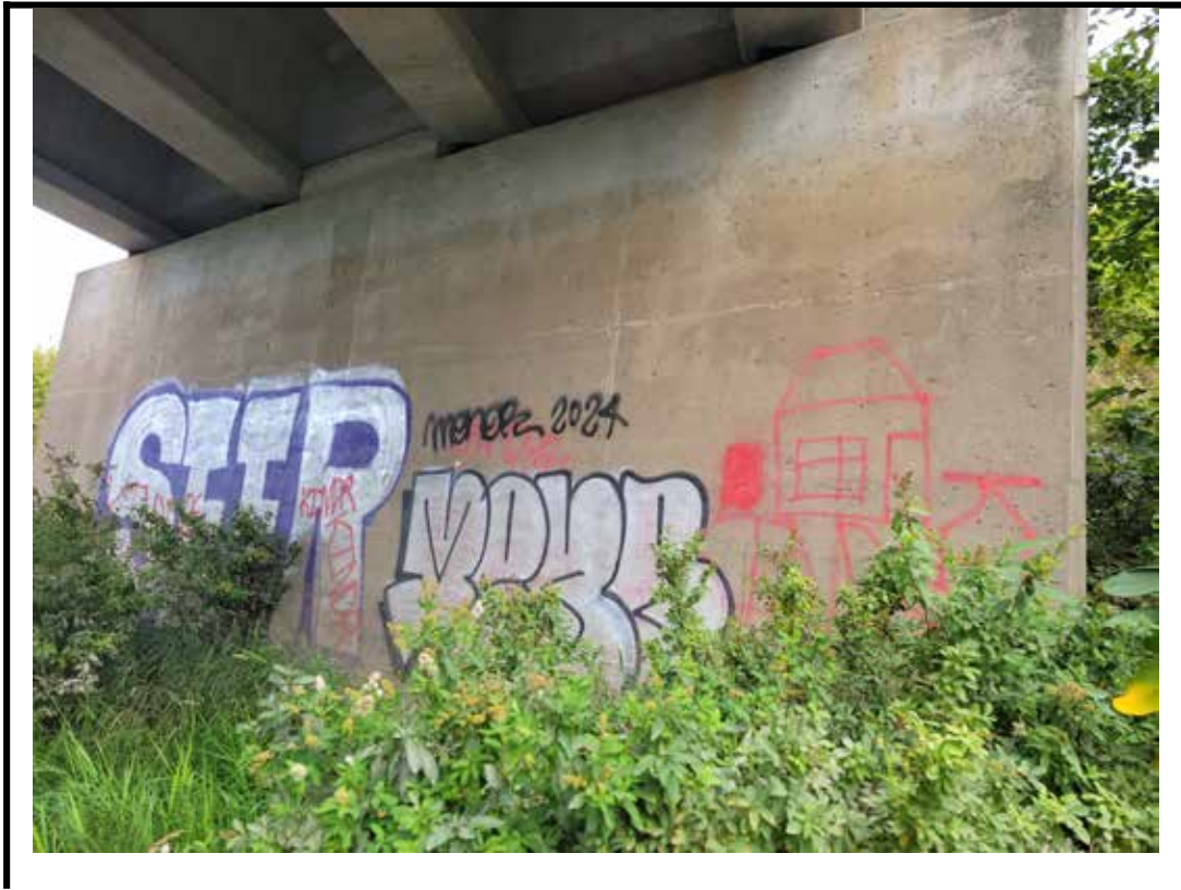
Photo 15 Graffiti on abutment walls
