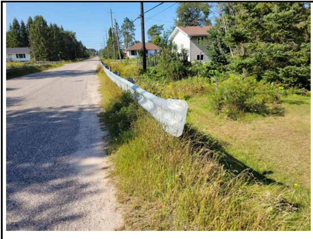
Photo 8 Vegetation overgrowing approach guide rail
