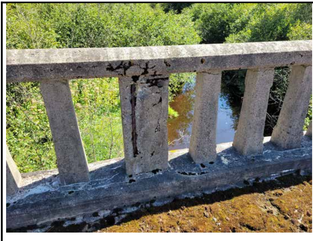
Photo 9 Spalls with exposed corroded reinforcement on concrete barrier
