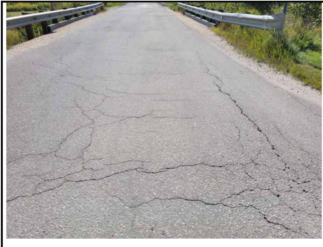
Photo 8 Medium and wide cracks on approach wearing surface
