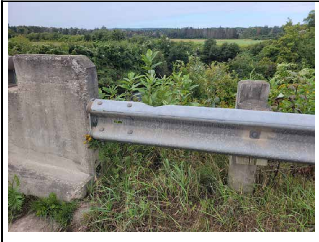
Photo 9 Substandard guide rail connection to deck barrier
