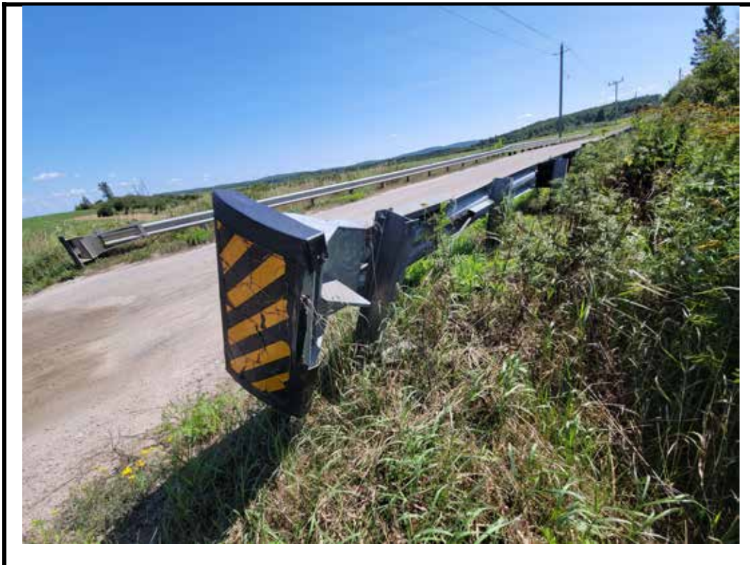
Photo 8 End treatment on northwest corner leaning and appear damaged
