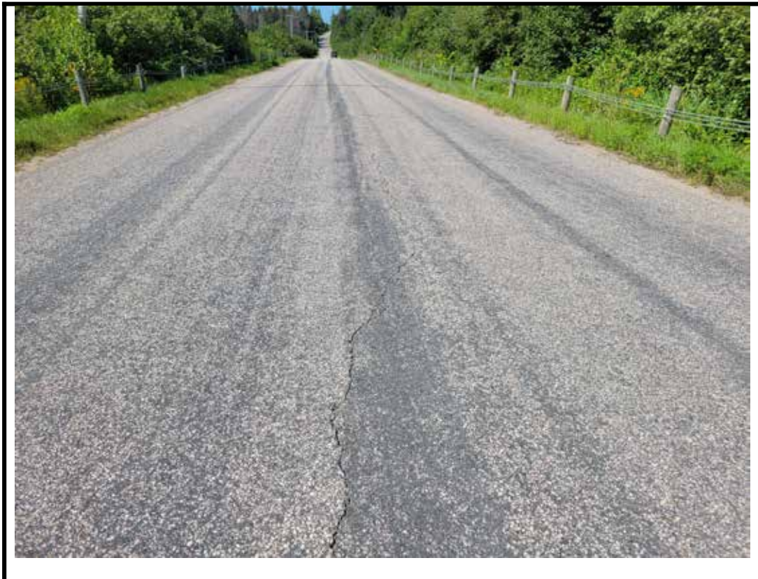
Photo 8 Longitudinal cracks along centreline on approach wearing surface
