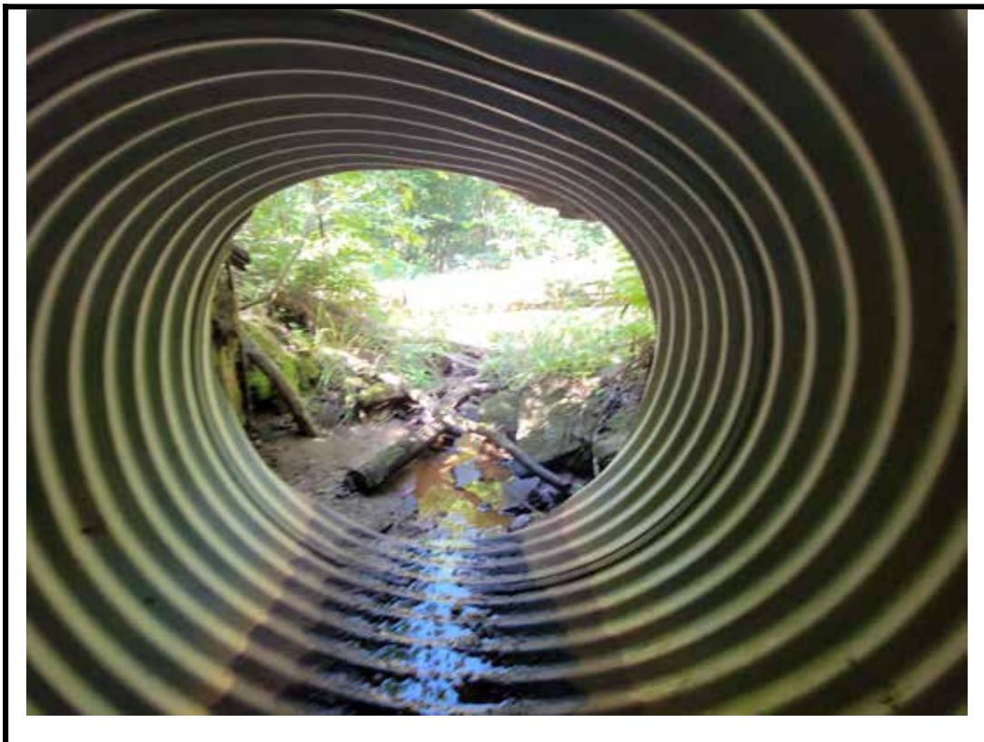
Photo 10 Deformation of north end of barrel
