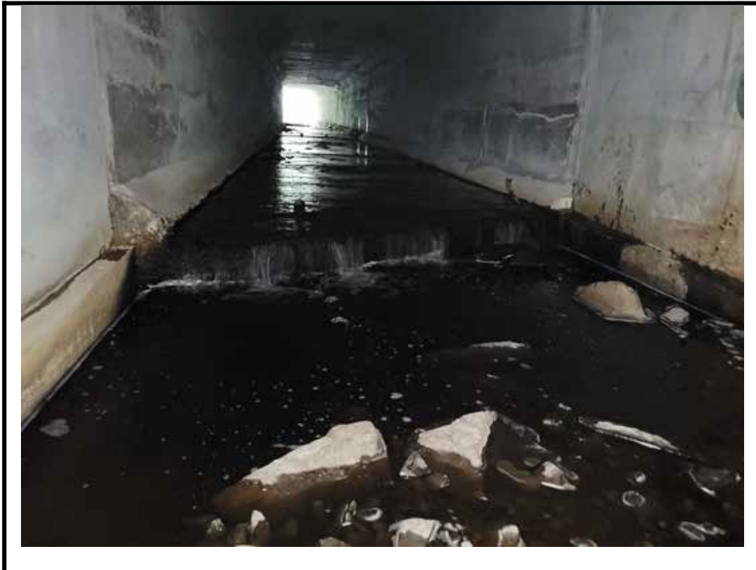
Photo 13 Drop in elevation of bottom slab at transition to west end section of barrel
