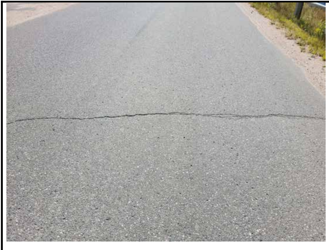
Photo 8 Transverse crack on east approach wearing surface
