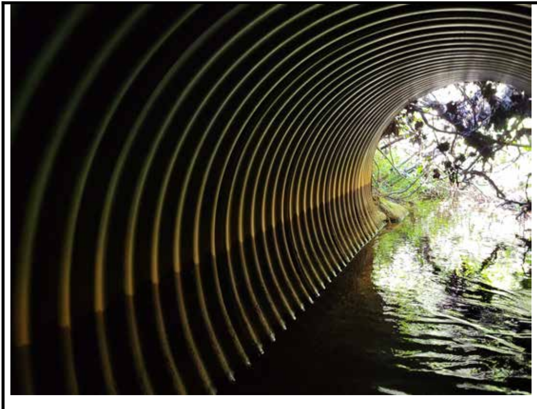
Photo 8 Light to moderate corrosion below the high water line throughout barrel
