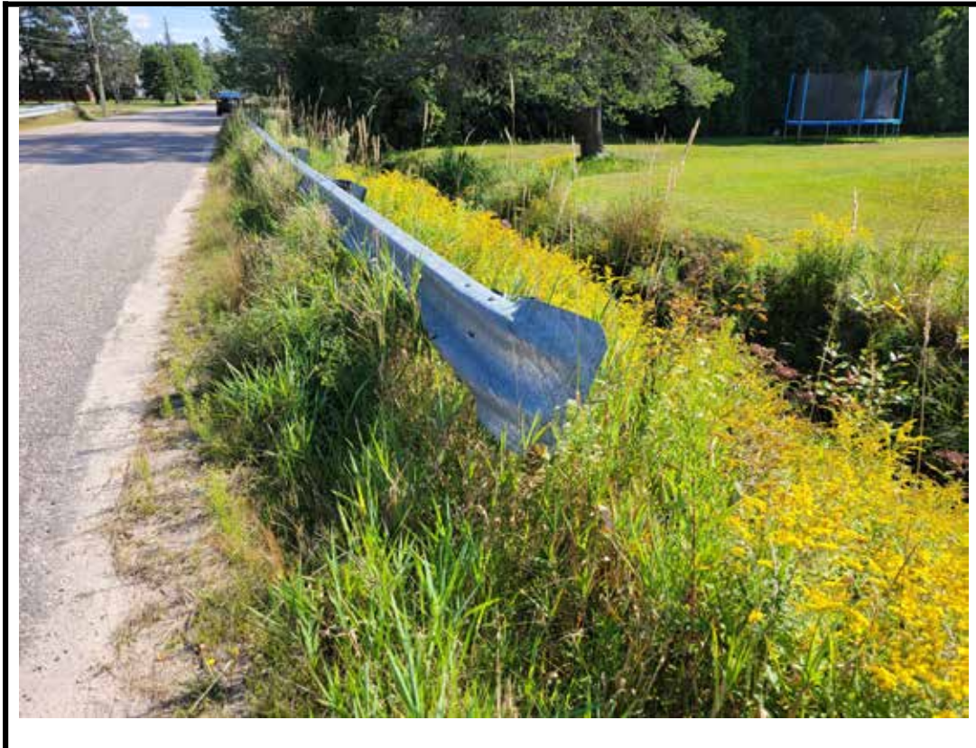
Photo 7 Substandard barrier and end treatment
