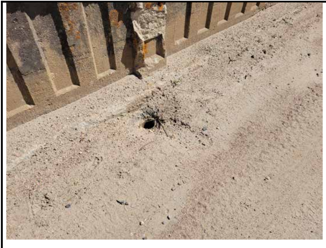
Photo 10 Accumulation of gravel throughout deck top
