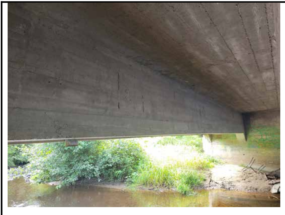
Photo 14 Small spalls with exposed corroded reinforcing steel on interior girder
