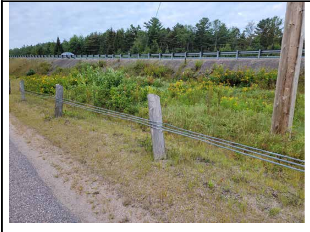
Photo 7 Substandard approach guiderail with loose cables
