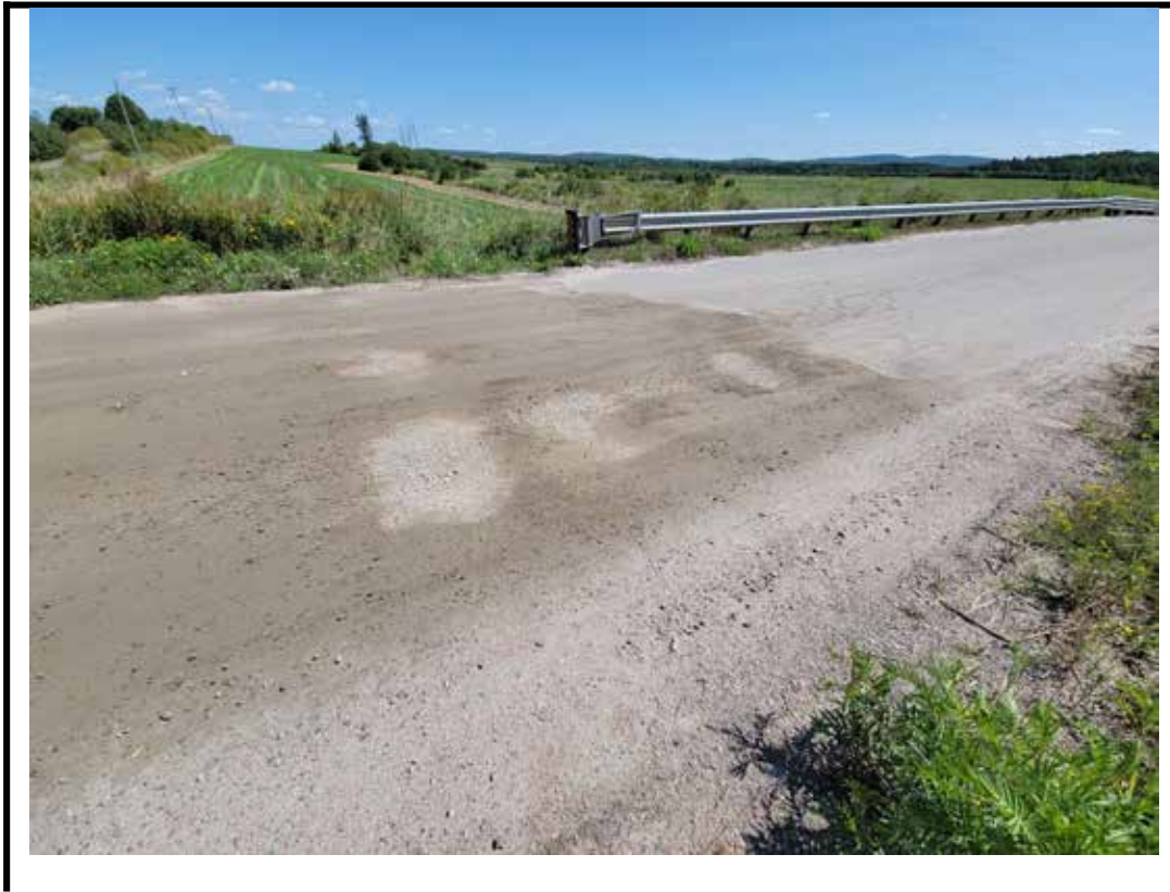
Photo 7 Potholes observed on north approach wearing surface
