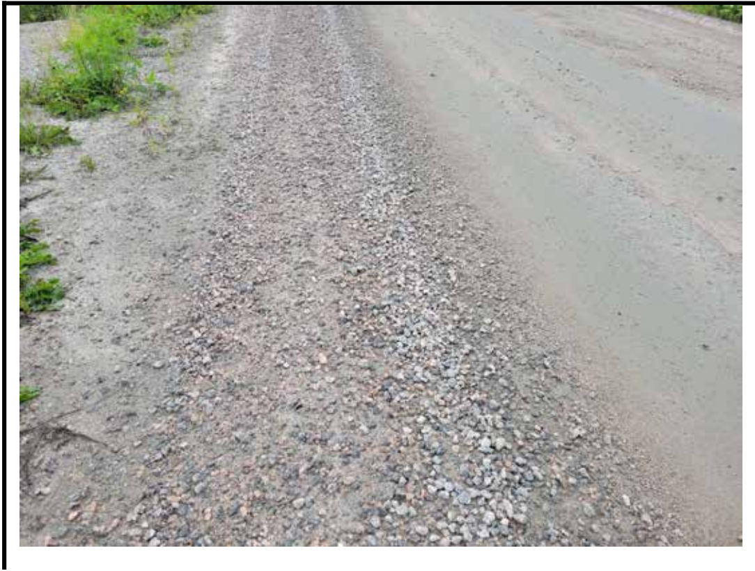
Photo 7 Loose gravel on wearing surface
