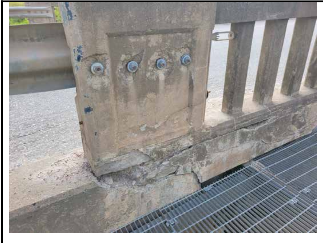
Photo 9 Localized spalls and concrete deterioration on west fascia
