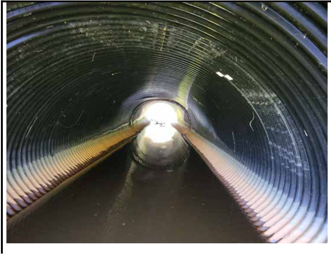
Photo 7 Light corrosion below the high waterline throughout the barrel
