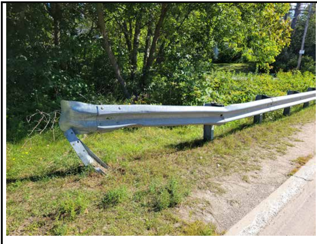
Photo 8 Impact damage on NW approach guide rail end treatment
