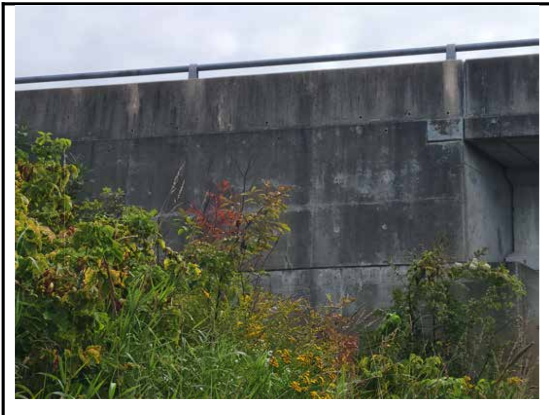
Photo 16 Weathering and narrow cracks on wingwall
