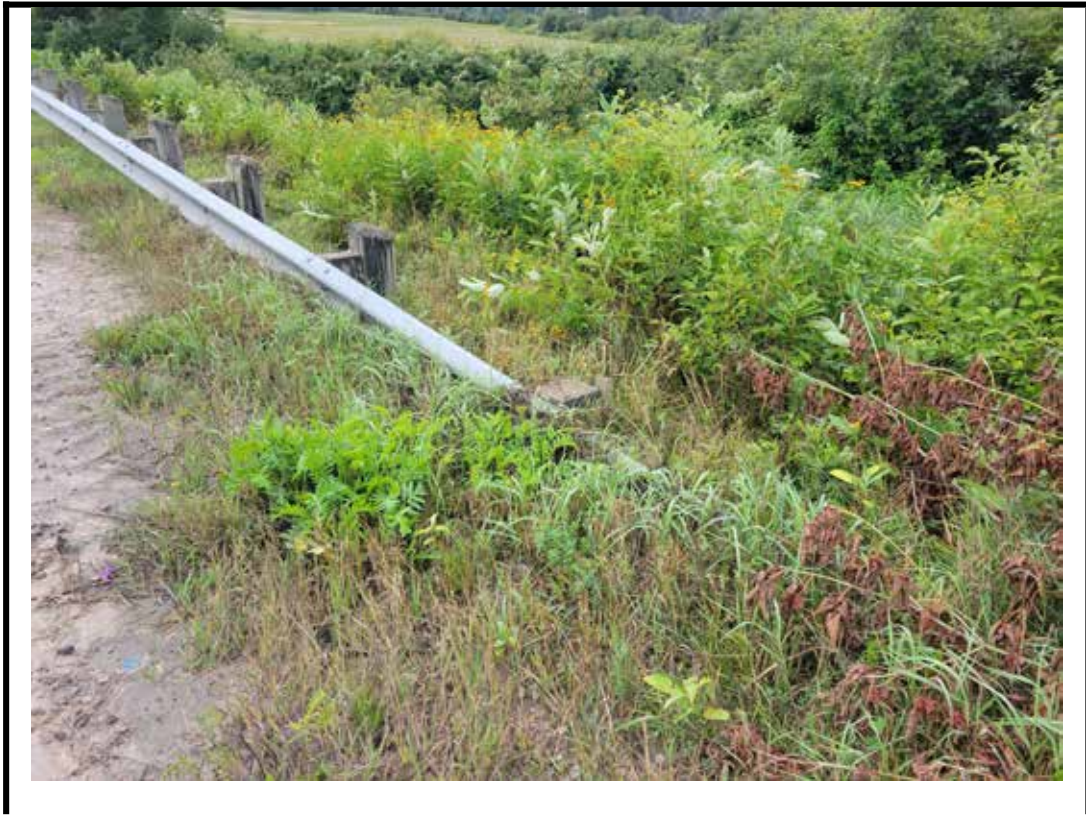
Photo 7 Substandard end treatment on NW approach guide rail
