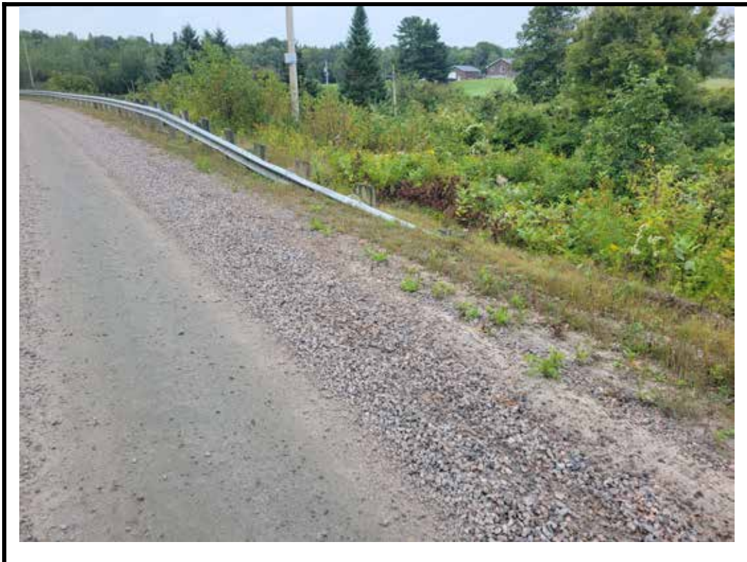
Photo 8 Substandard end treatment on NW approach guide rail
