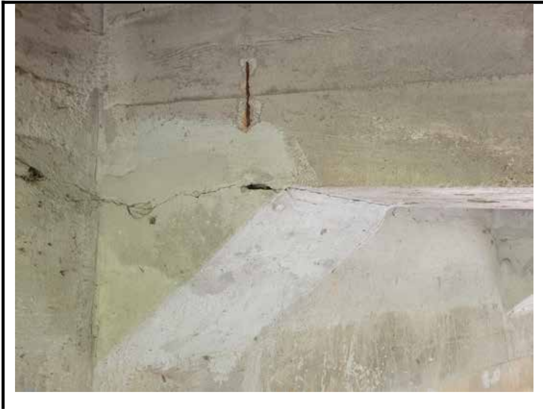
Photo 13 Medium horizontal crack and spall with exposed corroded reinforcing steel on girder
