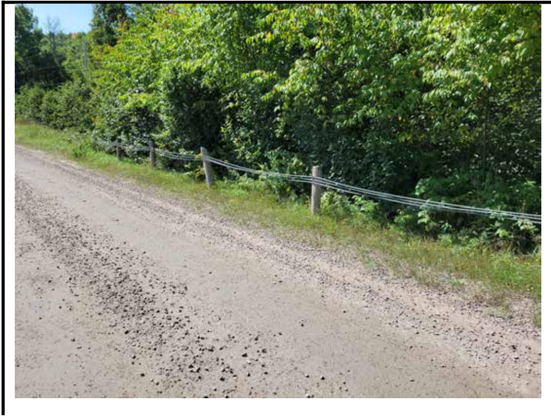
Photo 9 Loose guide rail cables
