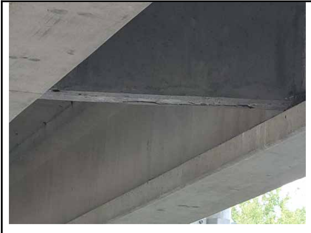
Photo 15 Cracks and delaminated concrete on underside of concrete diaphragms
