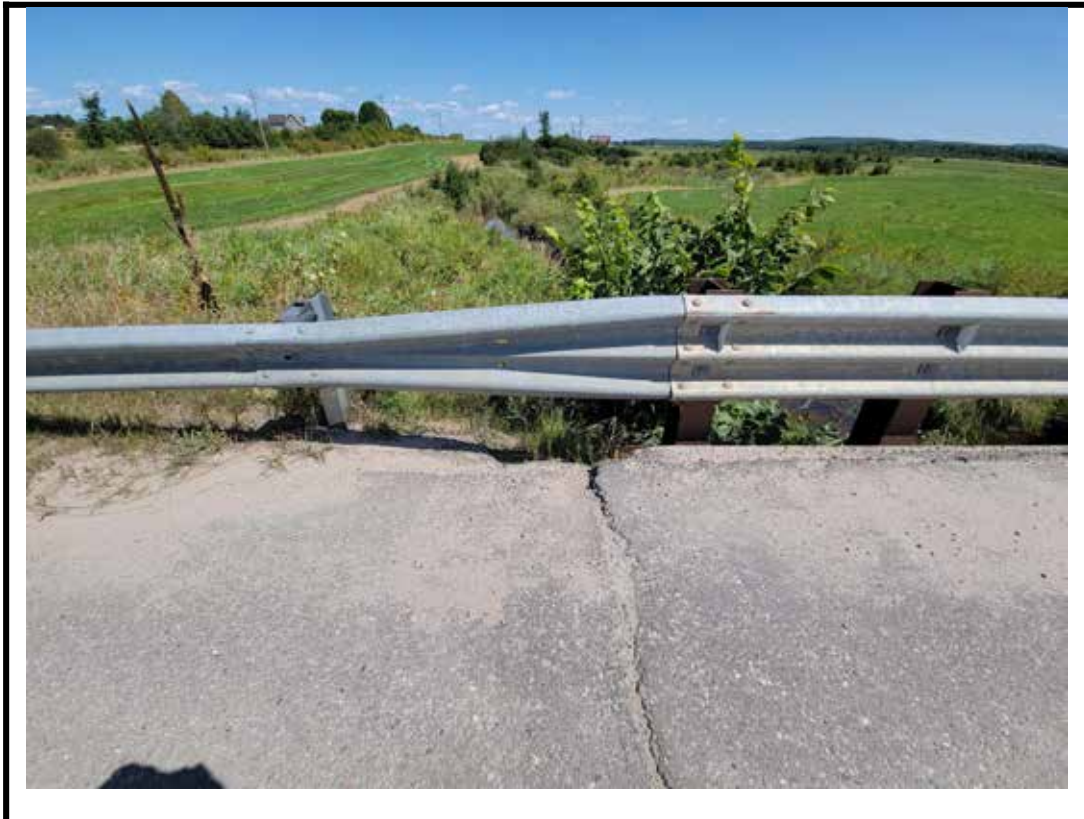
Photo 10 Missing guide rail post at transition rail to deck barrier (NE shown)
