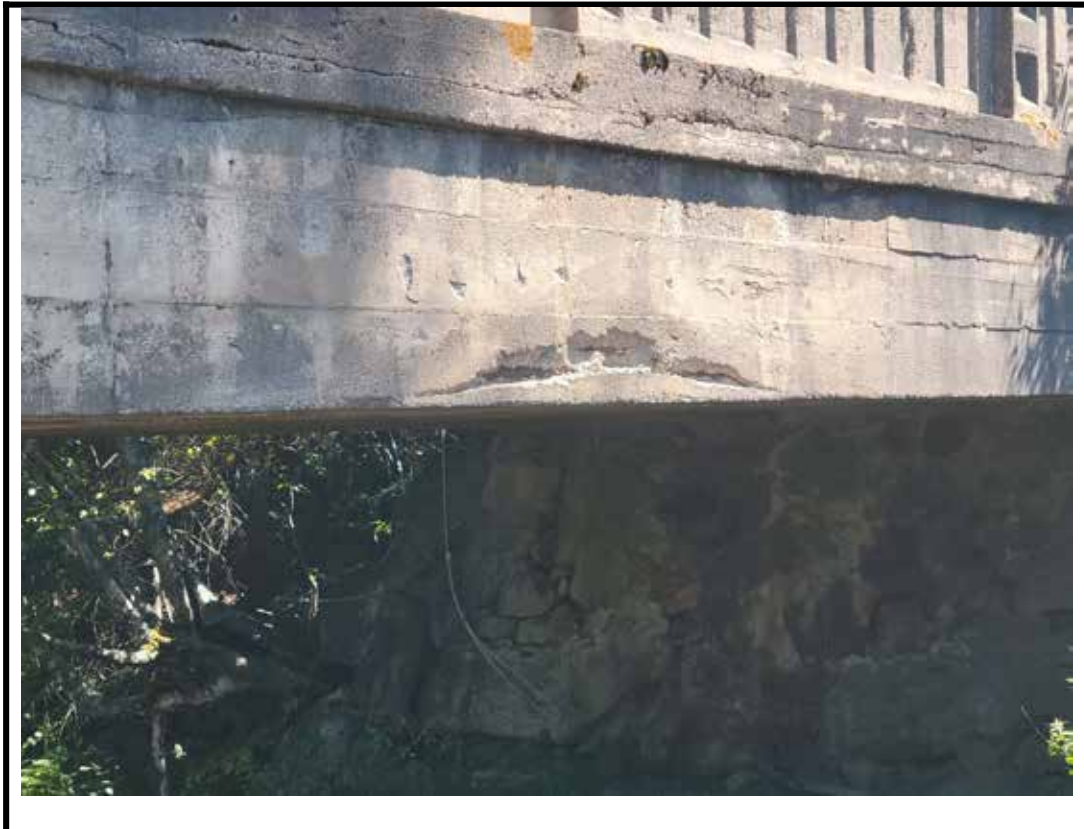
Photo 13 Spall and cracks on exterior face of girder at west side
