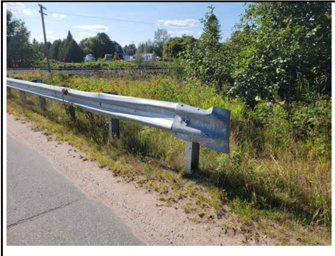
Photo 7 Deformation of northeast approach barrier end treatment
