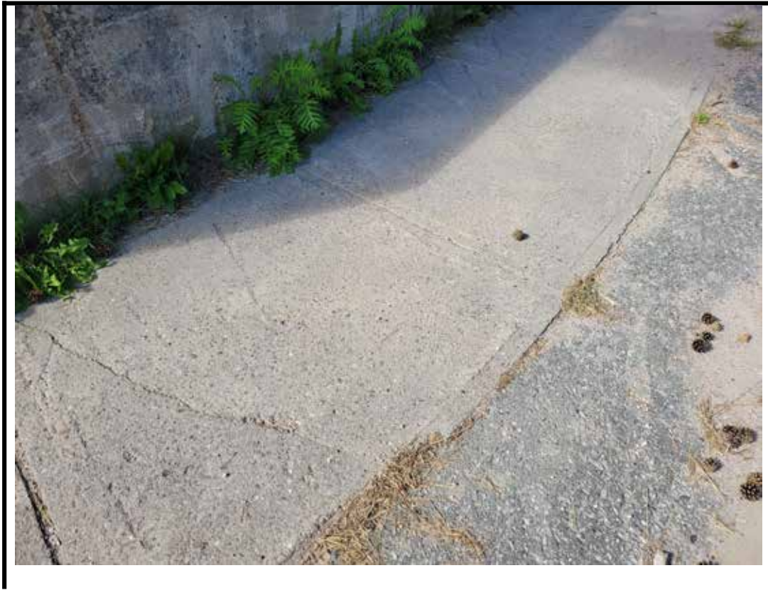
Photo 3 Medium transverse cracks and light to moderate scaling on sidewalk
