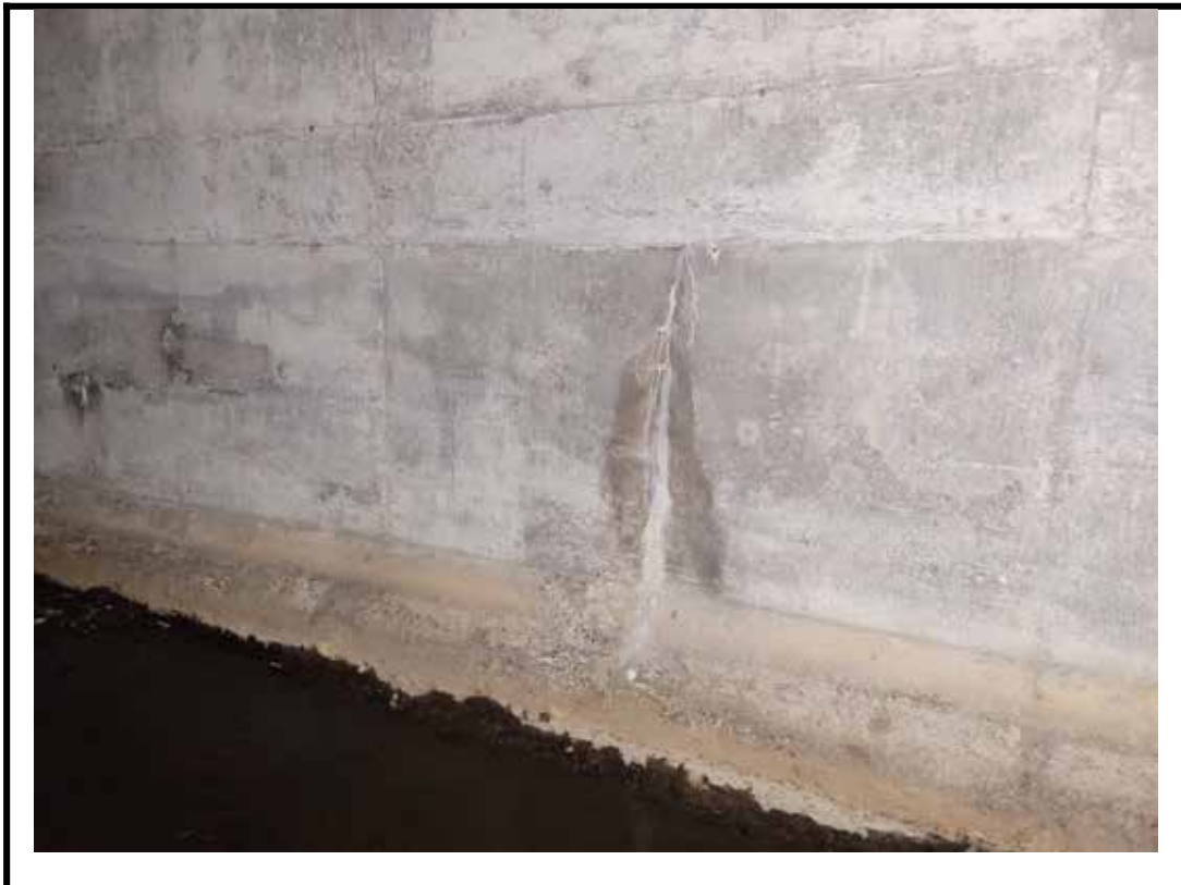
Photo 12 Narrow vertical cracks with efflorescence on north wall of barrel
