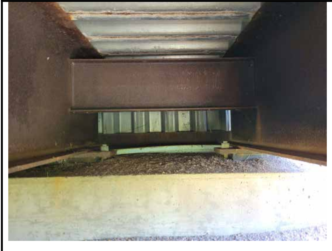
Photo 15 Debris accumulating on bearing seat
