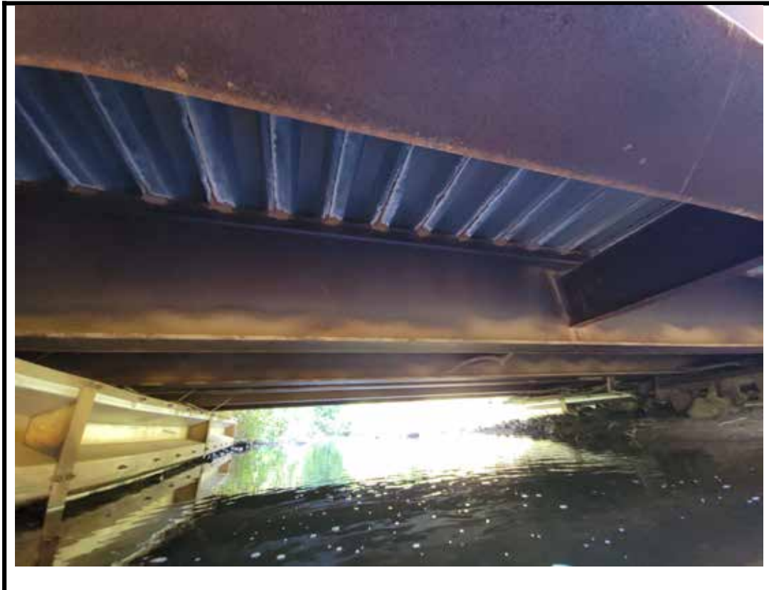
Photo 11 Light corrosion and efflorescence on v-pan soffit
