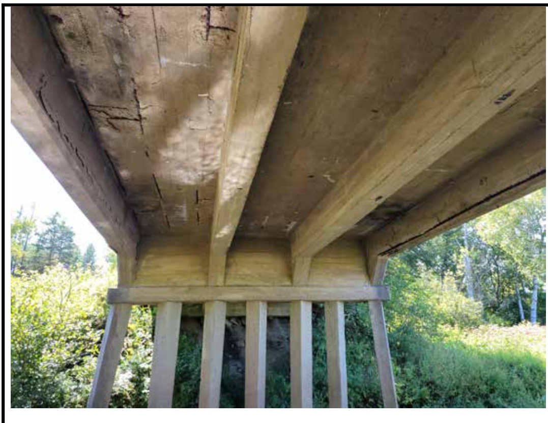
Photo 14 Efflorescence and damp staining on interior soffit of mid span
