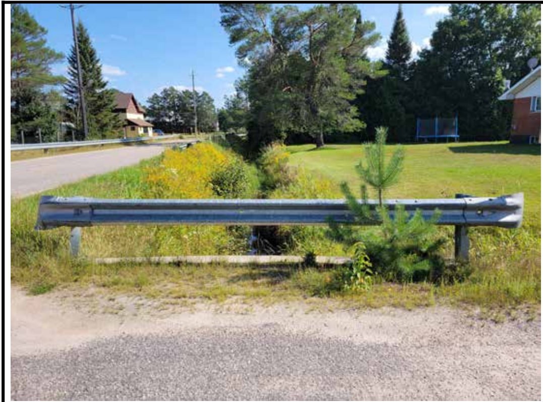
Photo 7 Substandard guiderail and end treatments over structure
