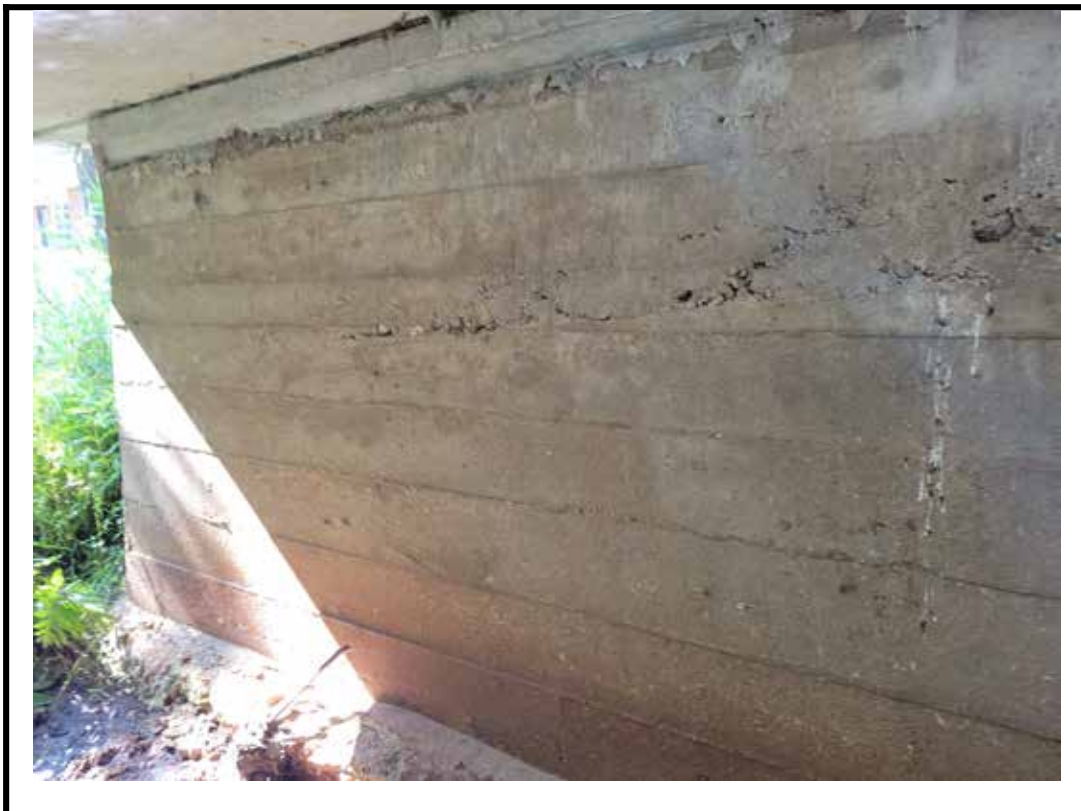
Photo 14 Isolated light honeycombing on north abutment
