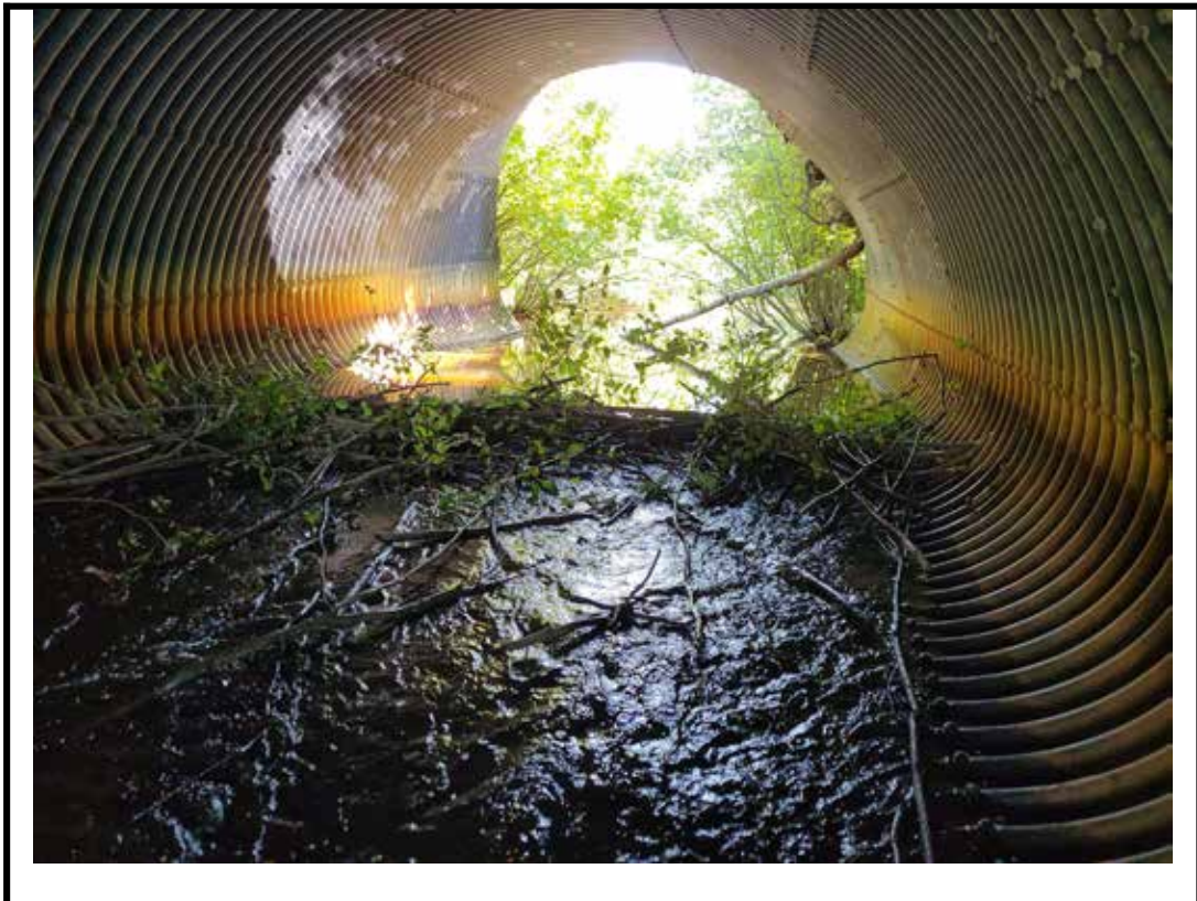
Photo 14 Accumulation of branches and debris causing restricted flow in barrel
