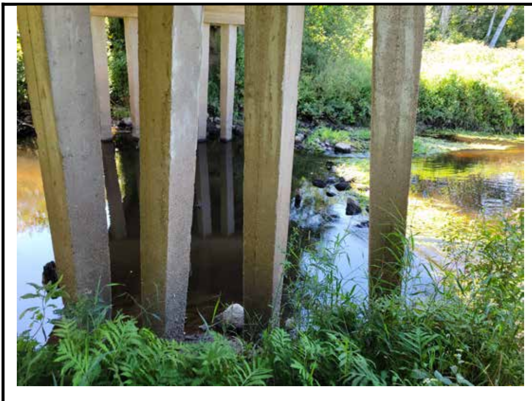
Photo 13 Light scaling and scouring on piers at waterline
