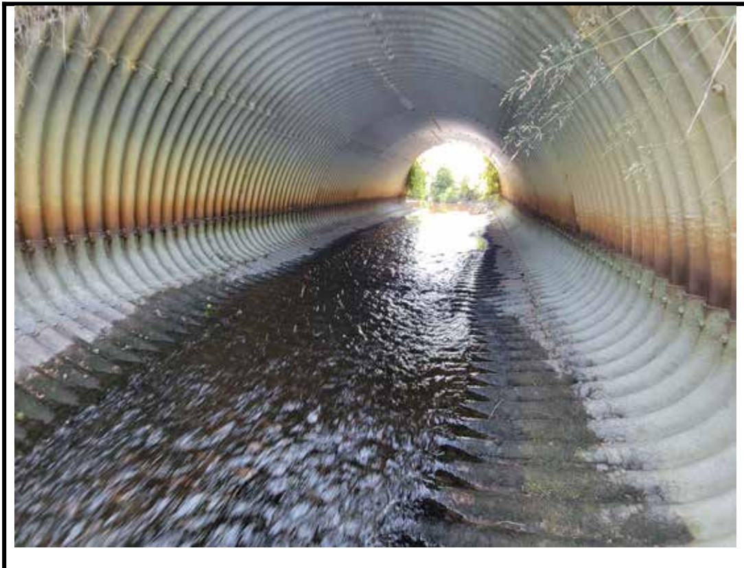
Photo 10 Light to moderate corrosion below the high water line throughout barrel
