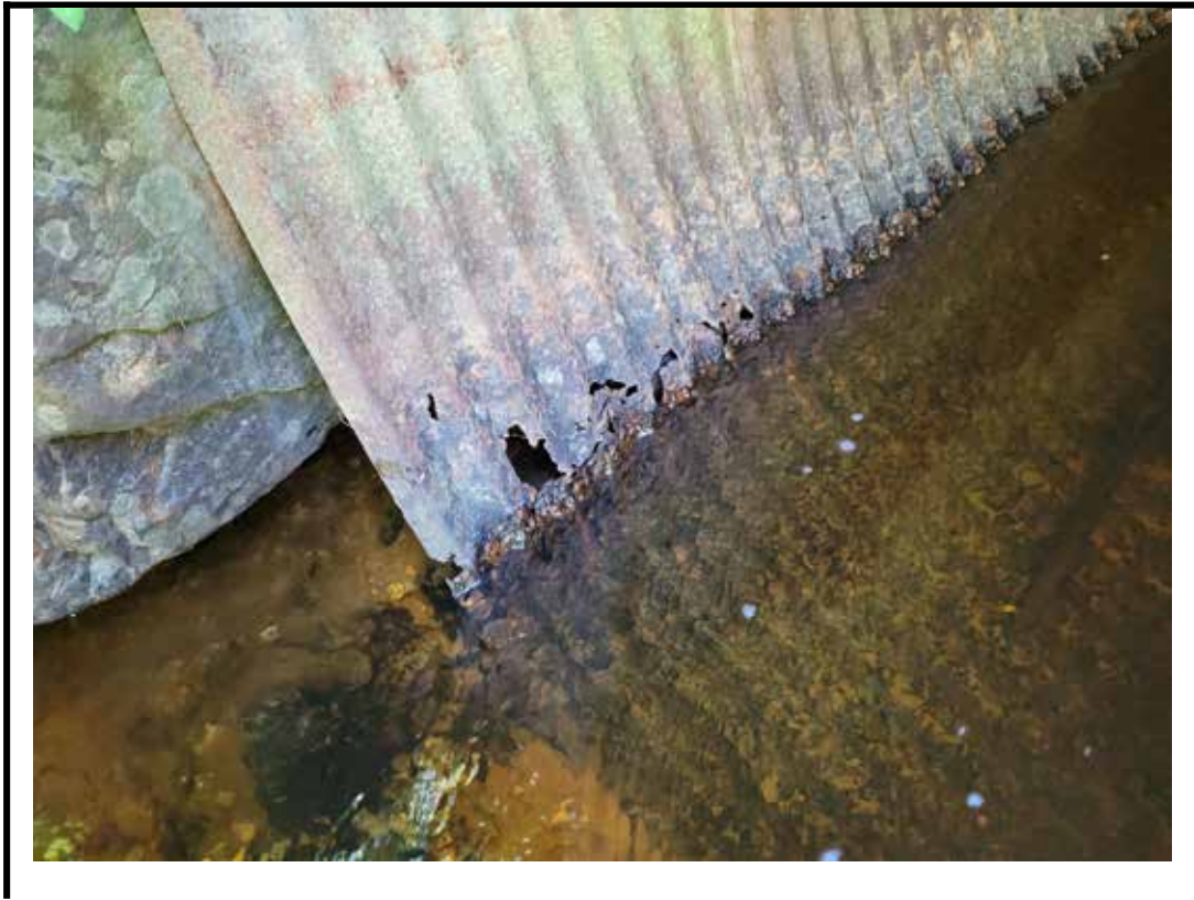
Photo 9 Moderate to severe corrosion of bottom of barrel with perforations at north end
