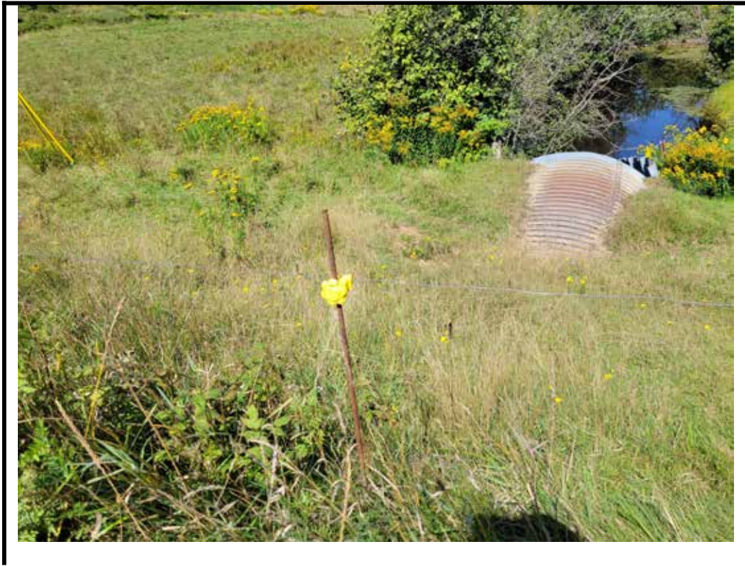
Photo 7 Electric fence present in north shoulder rounding beyond the gravel shoulder
