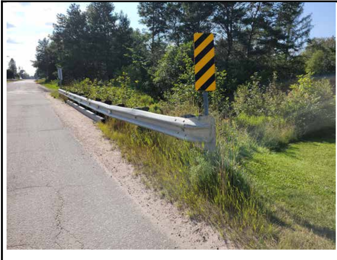
Photo 7 Substandard guide rail end treatment at NE corner of structure
