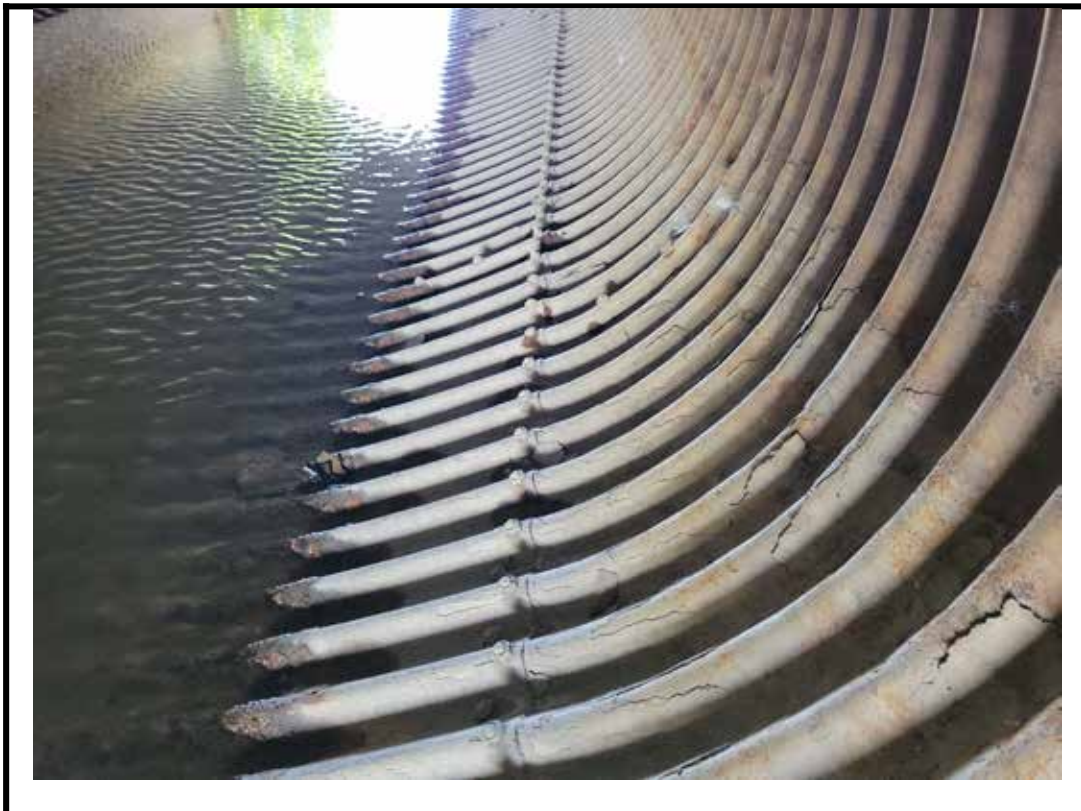
Photo 8 Light to localized moderate corrosion below the high water line
