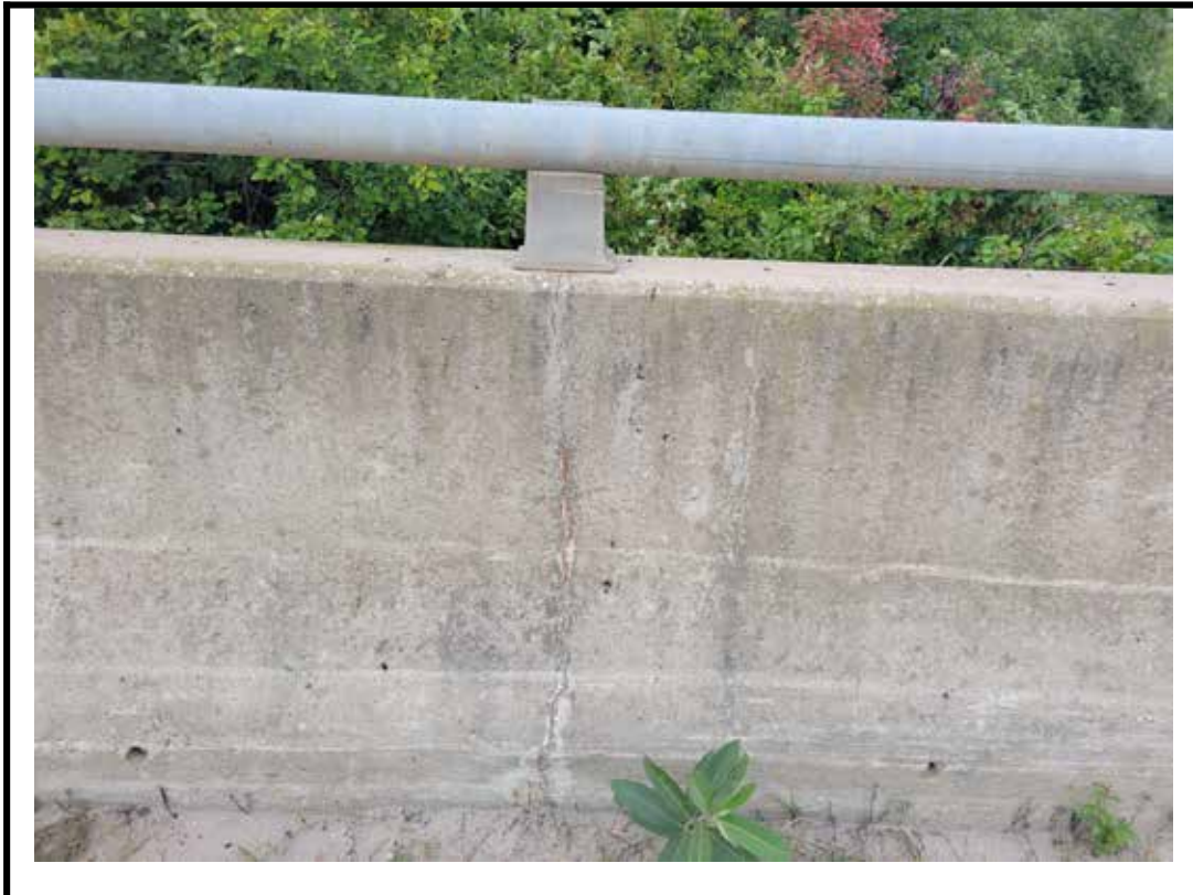
Photo 12 Narrow vertical cracks with damp staining on deck barrier
