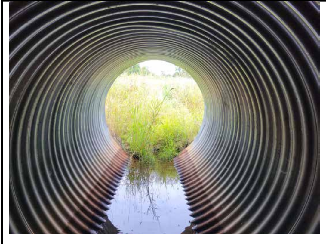
Photo 10 Vegetation encroaching into barrel at west end
