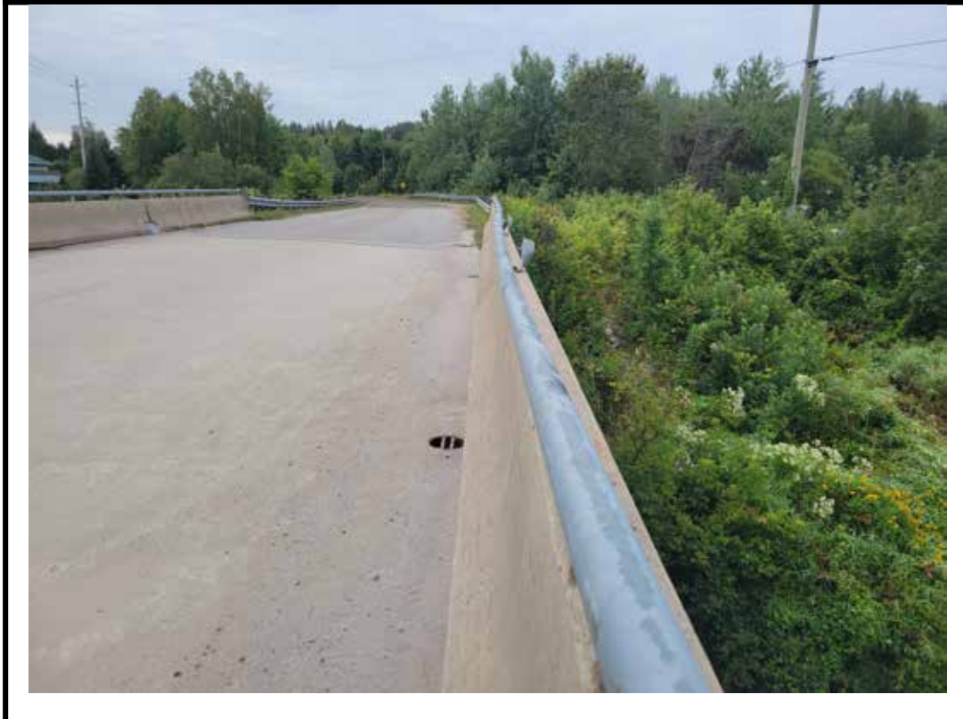
Photo 12 Severe damage and deformation of hand rail and posts on west side of structure
