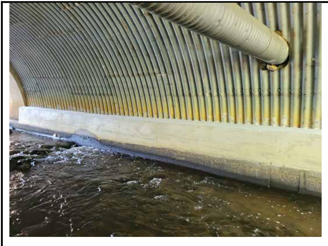
Photo 14 Light rust staining of barrel below the high water line
