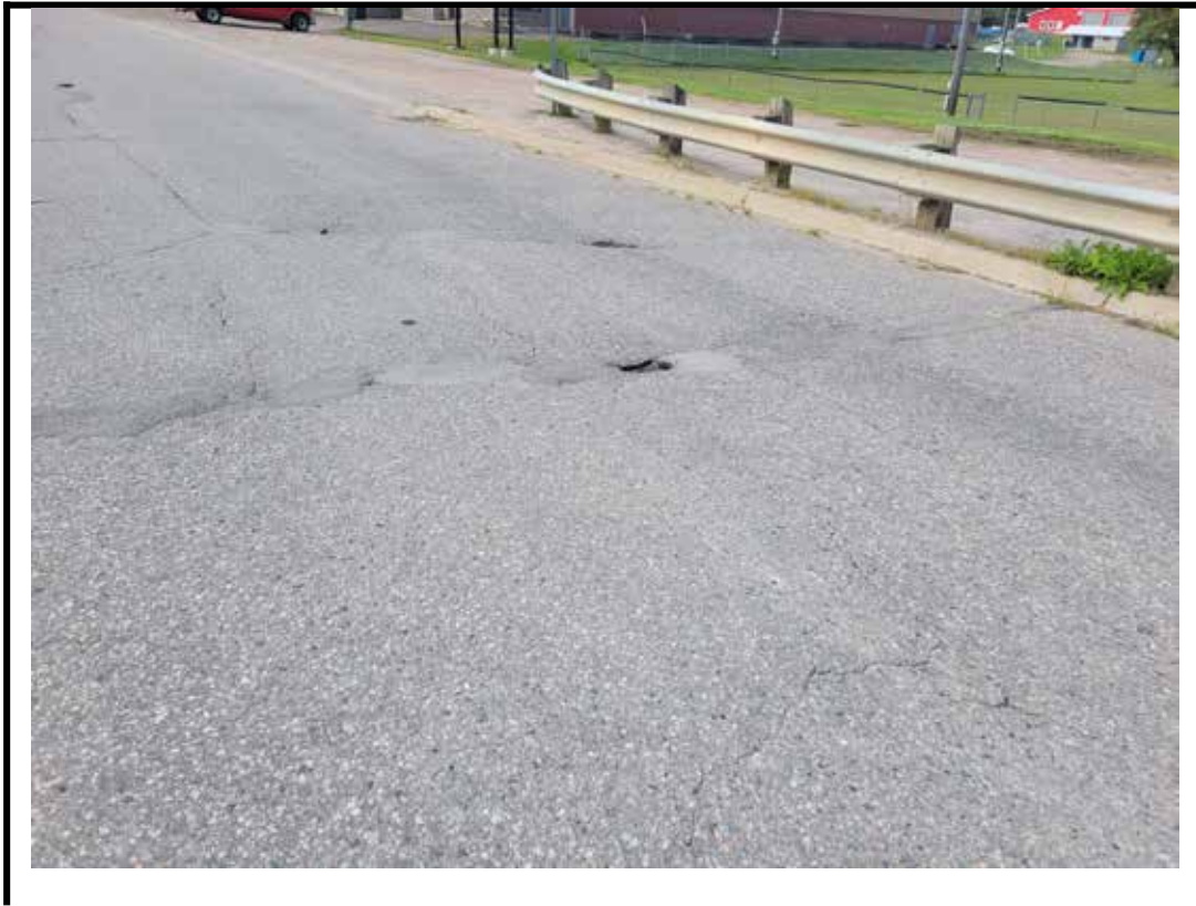
Photo 7 Medium to wide cracks and small potholes on south approach wearing surface
