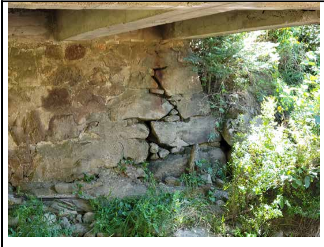
Photo 17 Wide cracks and mortar missing on south abutment wall
