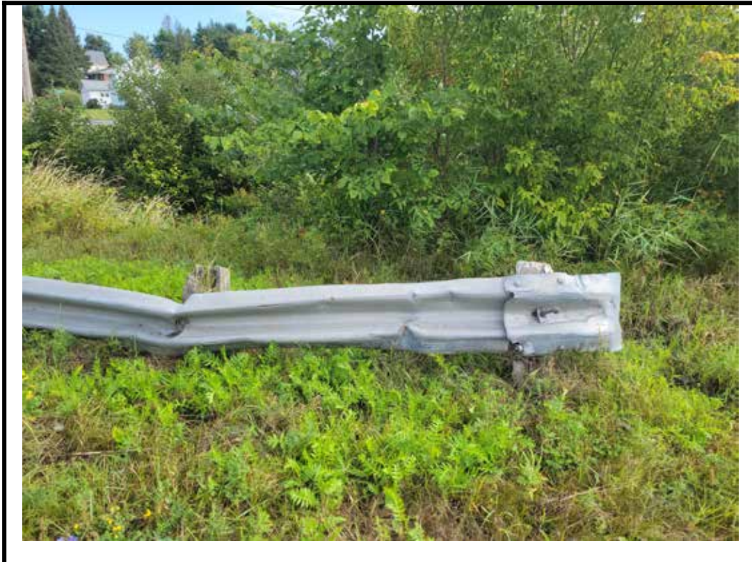
Photo 8 Substandard end treatment with severe deformations on SE approach guide rail
