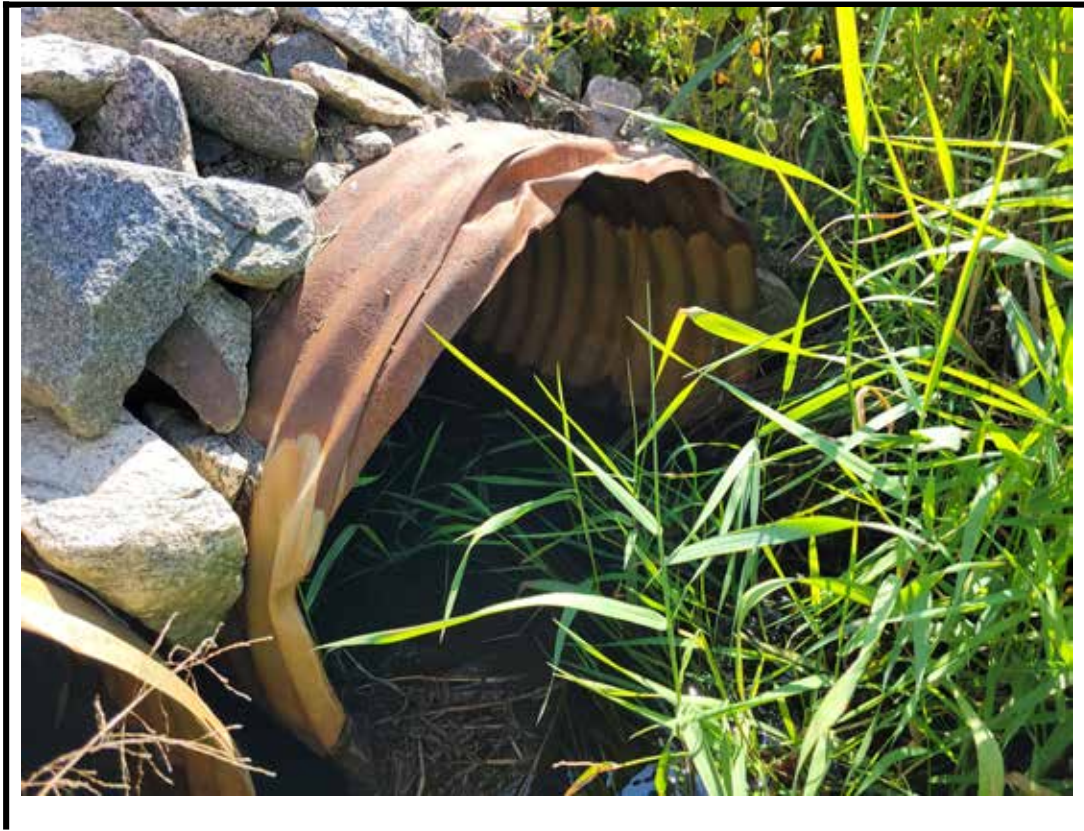
Photo 7 Damage at north end of west culvert barrel
