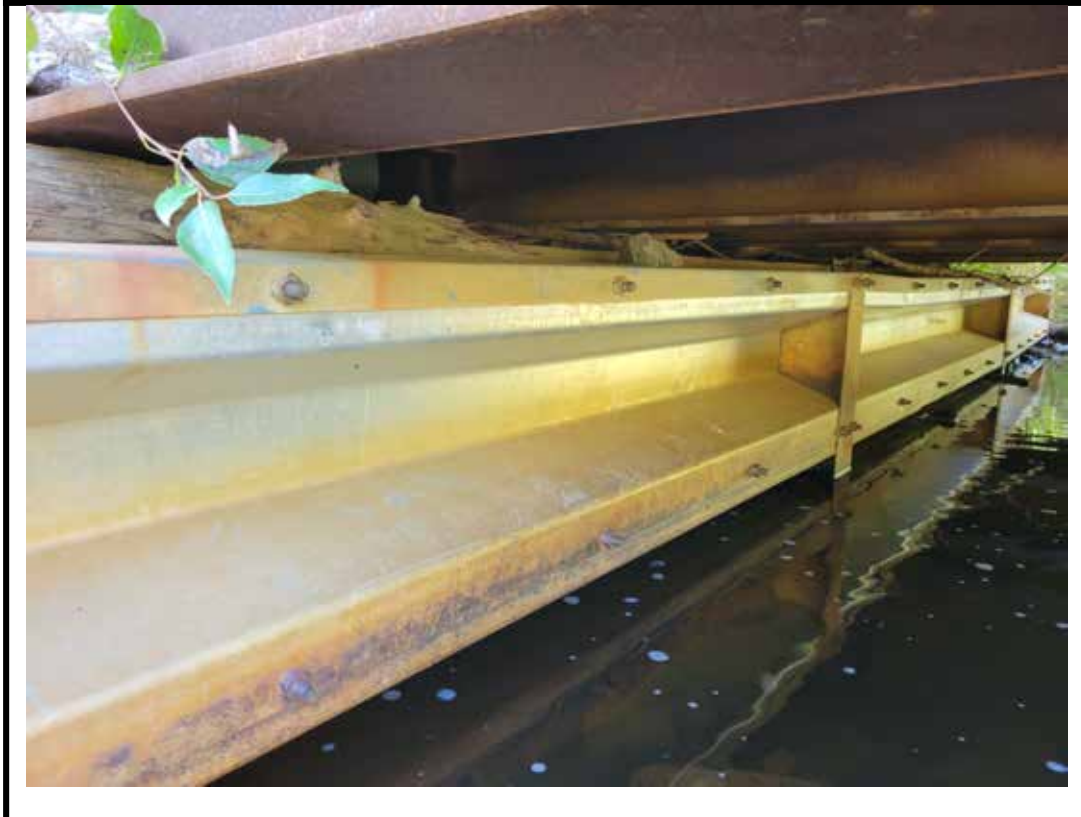
Photo 14 Light corrosion on west steel bin abutment at waterline
