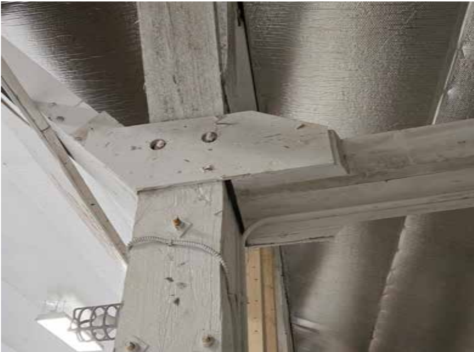
Photograph 5: Settlement effects at overhead structure
