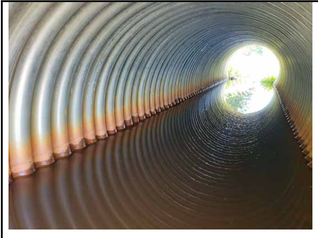
Photo 8 Light corrosion noted at waterline
