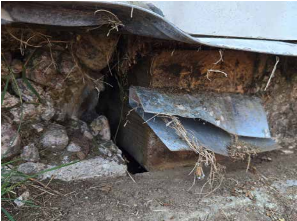
Photograph 7: Blocking at deteriorated column - exterior
