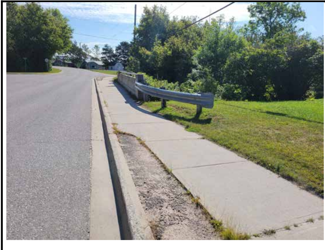
Photo 7 Substandard guiderail end treatment
