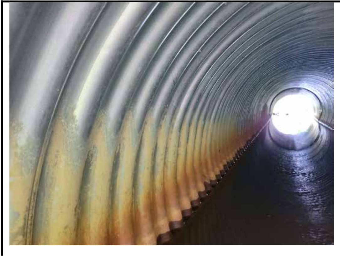
Photo 7 Light corrosion observed below the waterline
