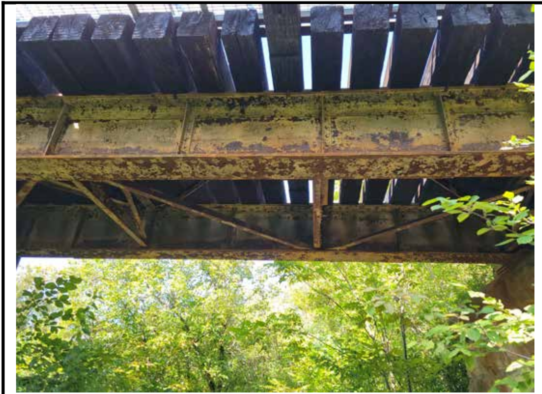
Photo 14 Coating failure and light to moderate corrosion of structural steel, north span
