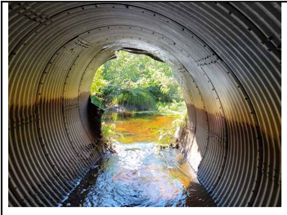
Photo 12 Deformations of south end of barrel
