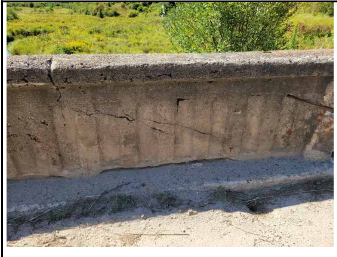
Photo 9 Small spalls, light to moderate scaling, and narrow to medium cracks on parapet
