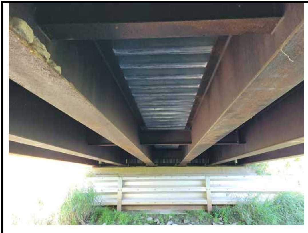
Photo 12 Localized light rust staining and light corrosion on girder and interior soffit
