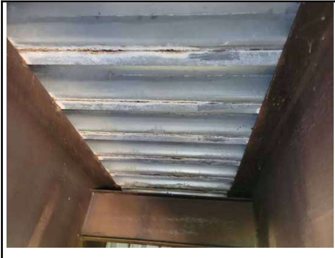
Photo 11 Light corrosion and efflorescence on steel deck soffit end
