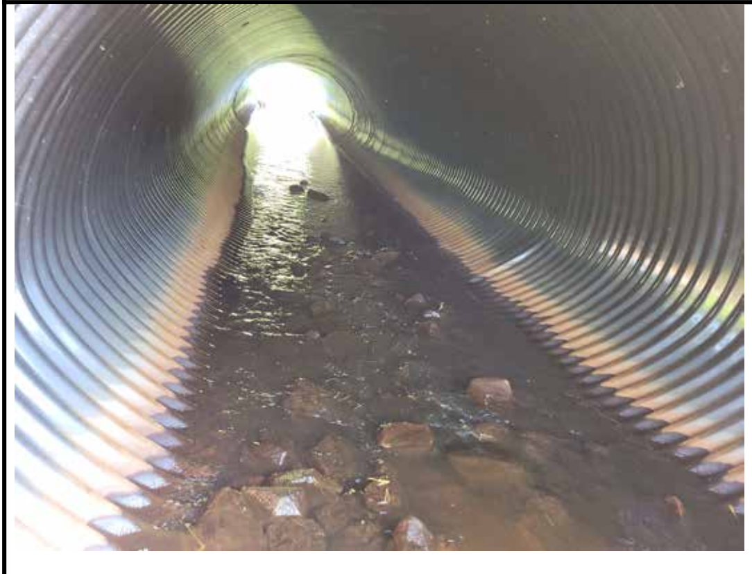
Photo 9 Rocks accumulating in west end of barrel
