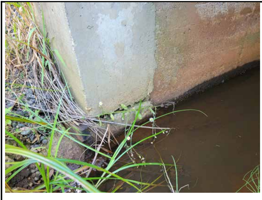
Photo 12 Wide crack in reconstruction at NE corner of barrel
