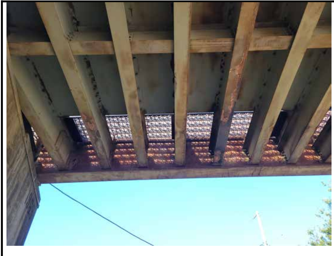
Photo 7 Light corrosion and coating failure on structure steel members
