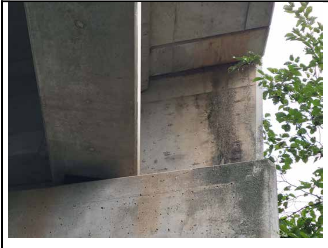
Photo 13 Damp staining on north ballast wall
