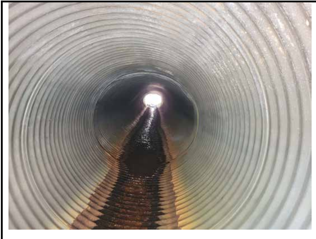
Photo 8 Light to moderate corrosion throughout bottom of barrel
