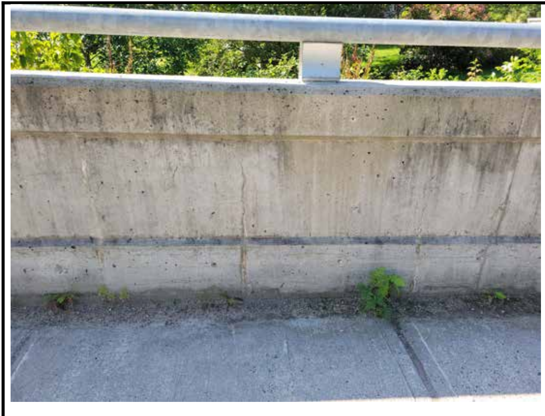
Photo 10 Narrow vertical cracks with efflorescence on concrete parapet wall
