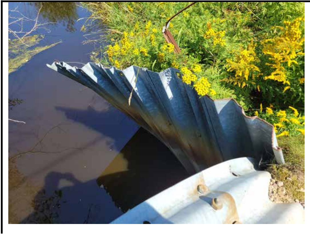
Photo 11 Deformation of sheet pile retaining wall
