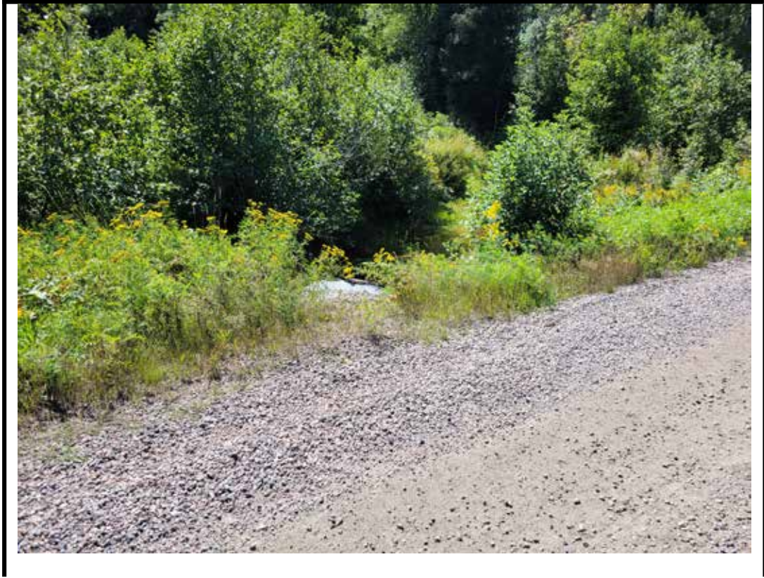
Photo 7 Loose gravel accumulating on edges of roadway
