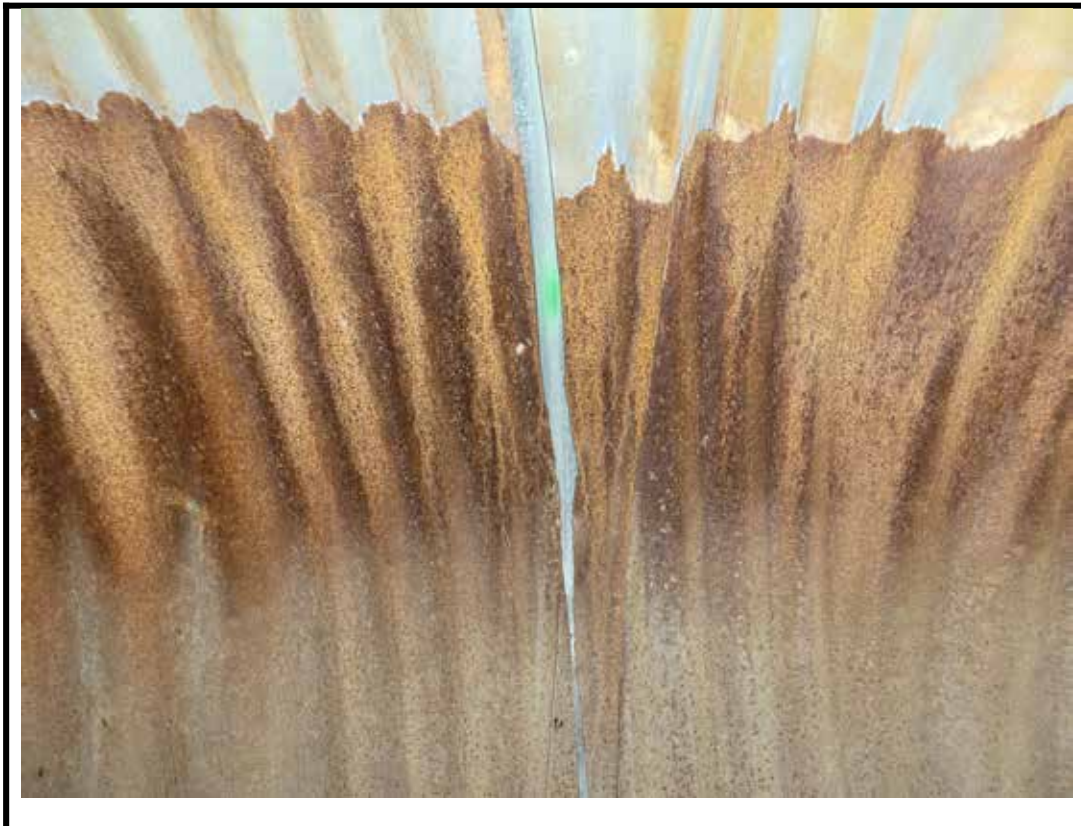
Photo 8 Joint separation forming inside barrel
