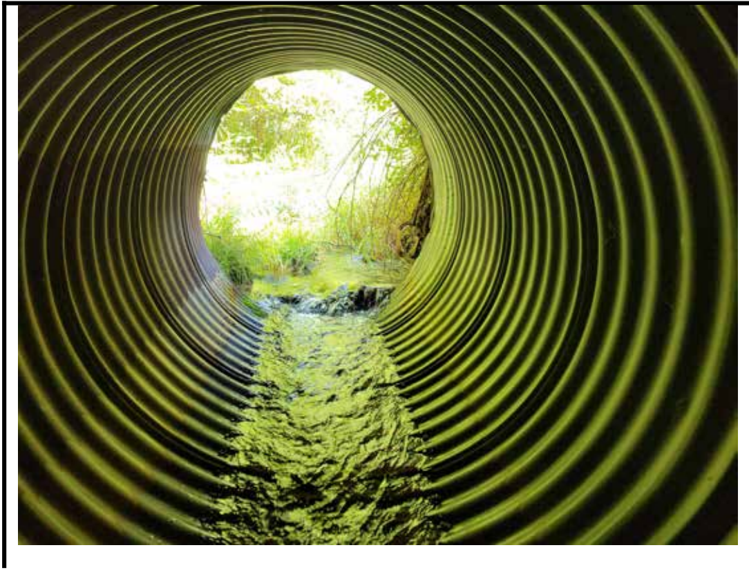
Photo 9 Small deformation noted inside barrel at west end
