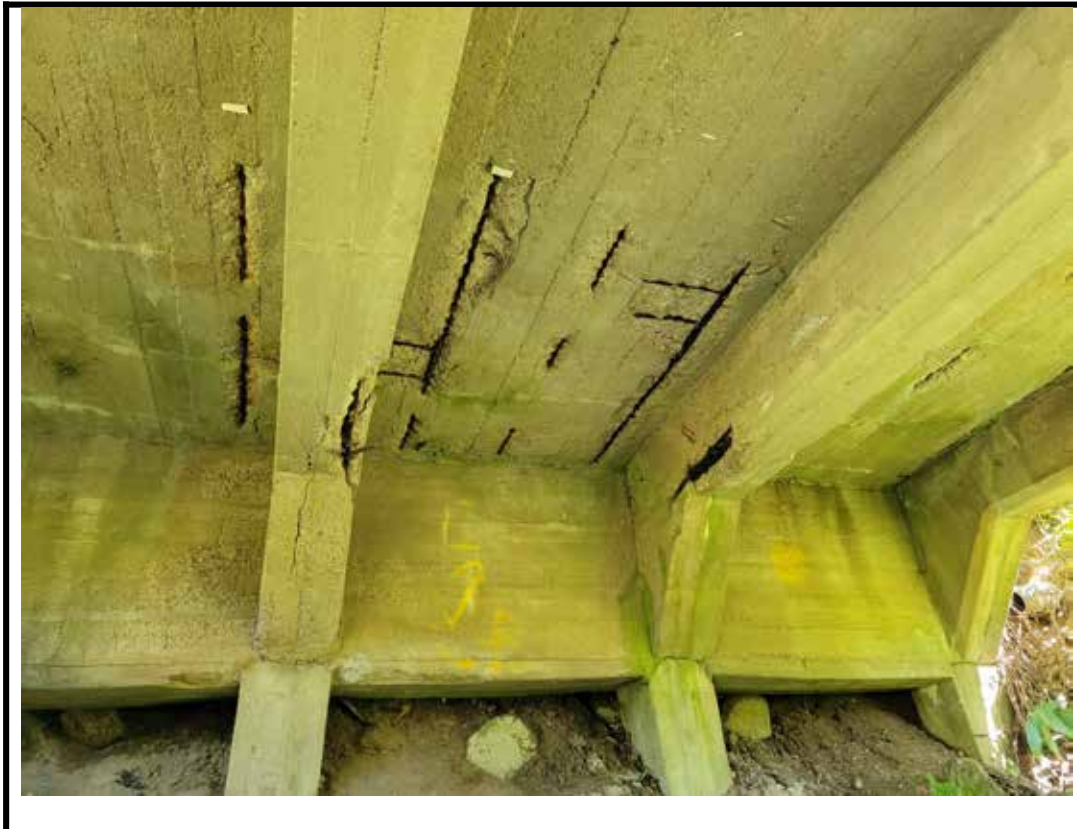
Photo 11 Severe spalls with exposed corroded reinforcing on north span girders and soffit
