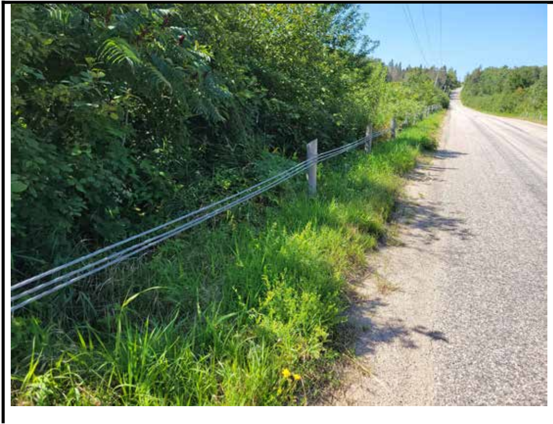
Photo 7 Substandard approach guide with loose cables
