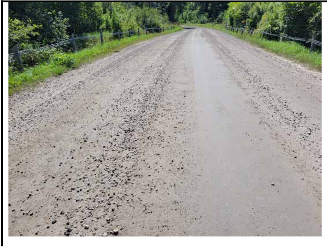
Photo 7 Small potholes and loose gravel on wearing surface
