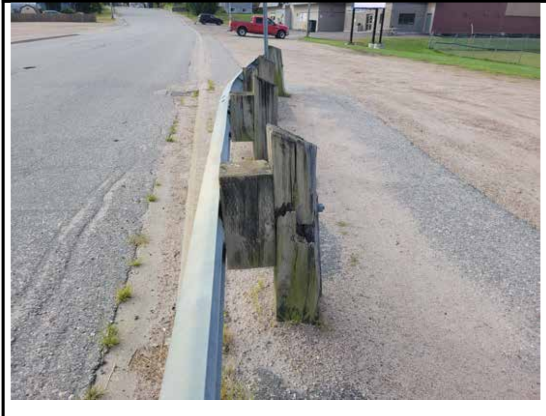
Photo 10 Damaged timber approach guide rail post on SW approach
