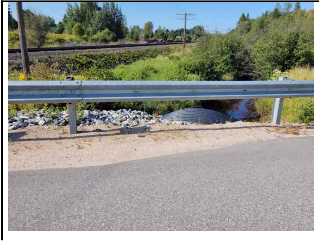
Photo 9 Missing barrier post over culvert barrel
