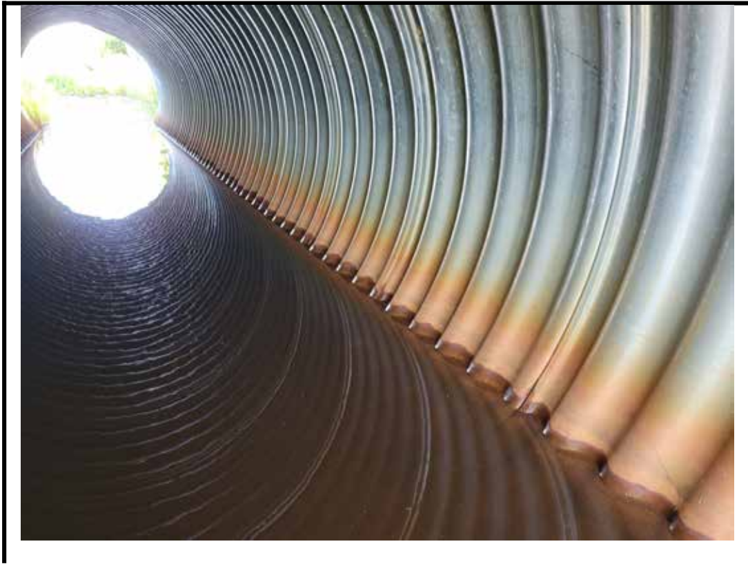
Photo 7 Light to severe corrosion noted along waterline
