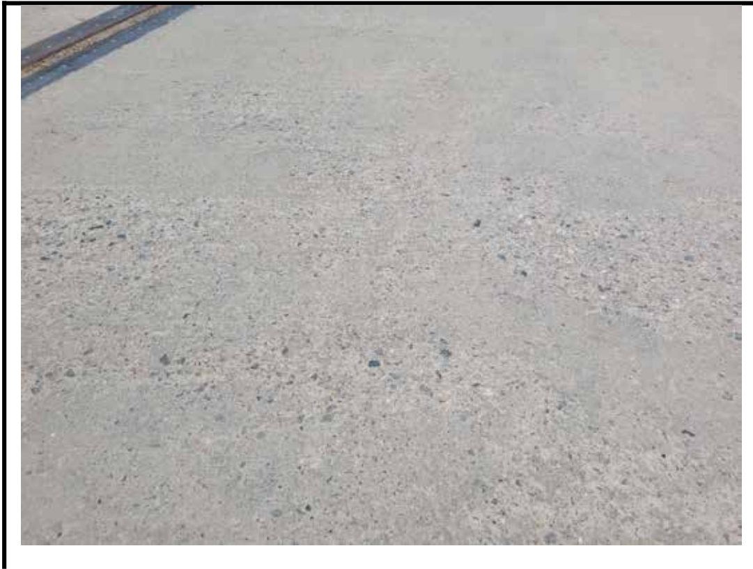
Photo 11 Light to localized moderate scaling on exposed deck top
