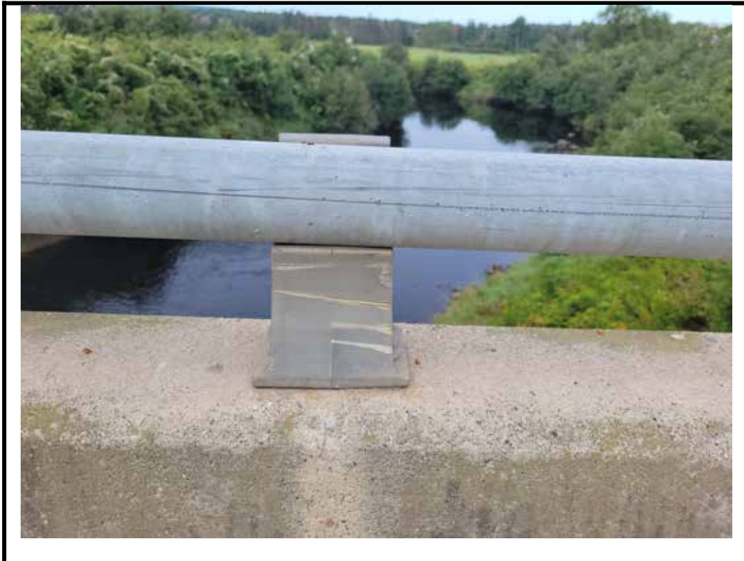
Photo 11 Deformation and abrasions on steel pipe hand rail post over west side of deck
