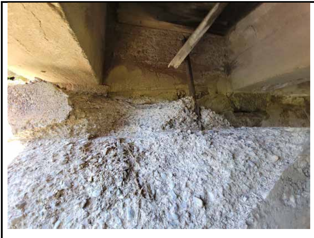
Photo 18 Disintegration at top of the north abutment wall, west end
