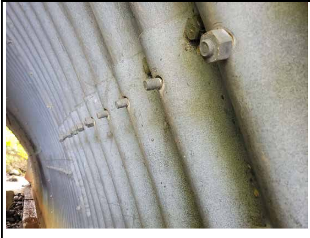
Photo 9 Missing nuts on steel plate bolted connections in barrel
