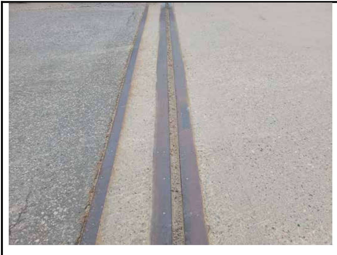
Photo 10 Light raveling on concrete end dams and end of exposed deck
