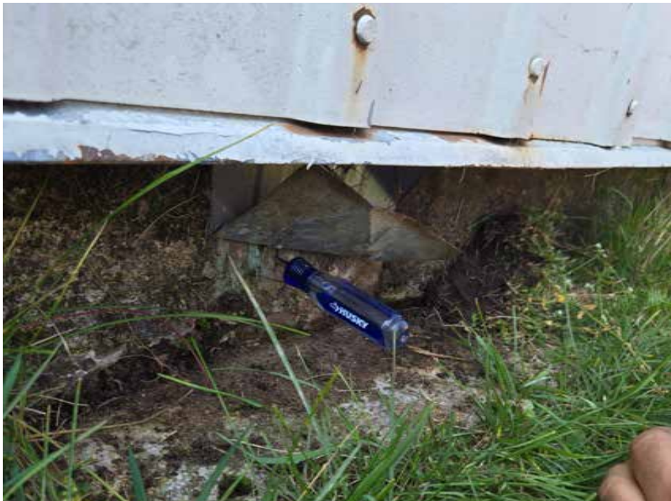
Photograph 6: Deterioration at original column - exterior
