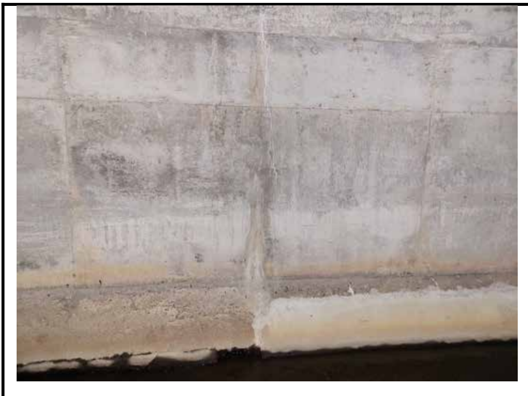
Photo 10 Light to localized moderate scaling and narrow vertical cracks with efflorescence on barrel wall
