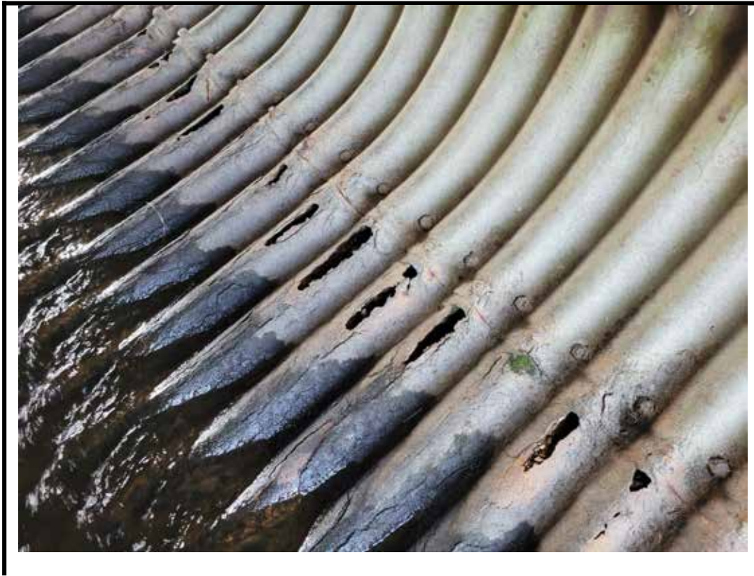
Photo 11 Localized severe corrosion with perforations in bottom of barrel
