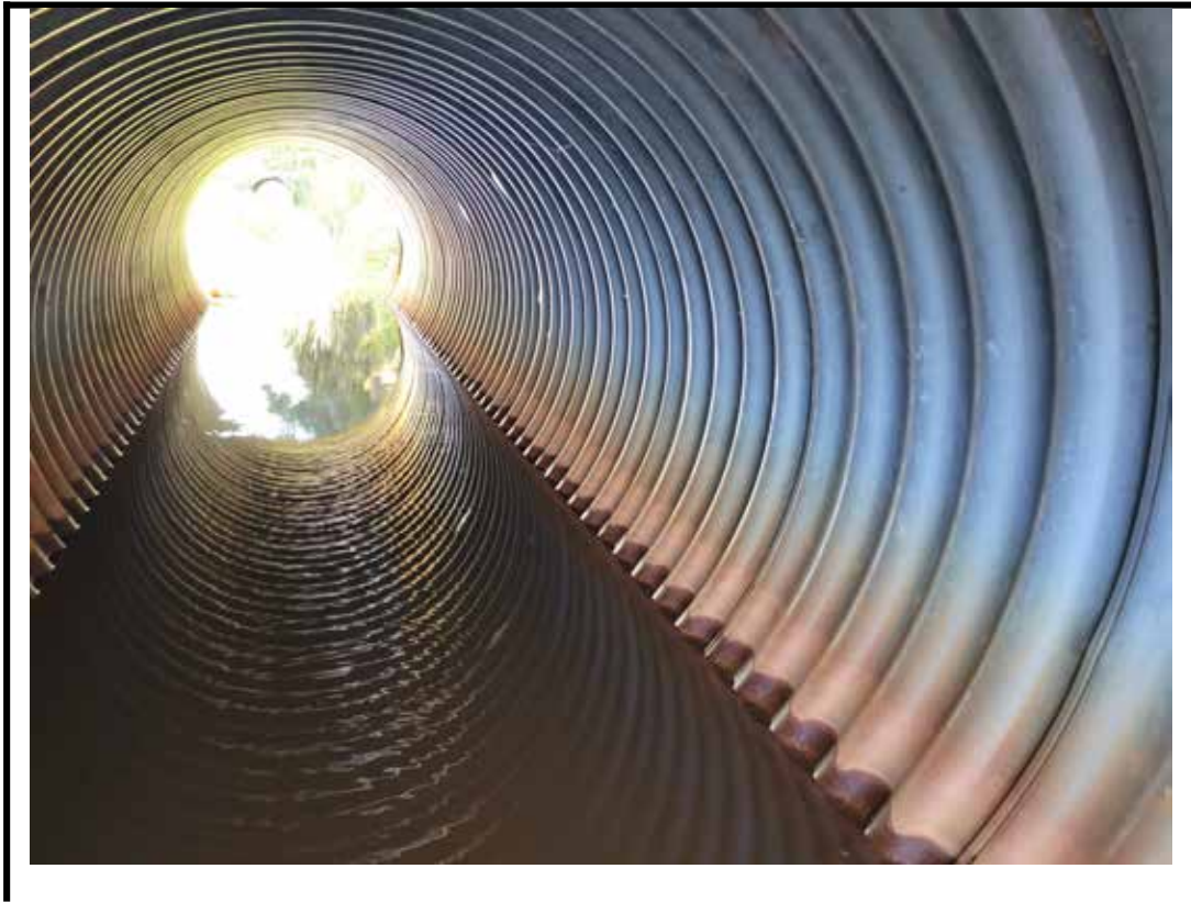
Photo 7 Light corrosion at waterline
