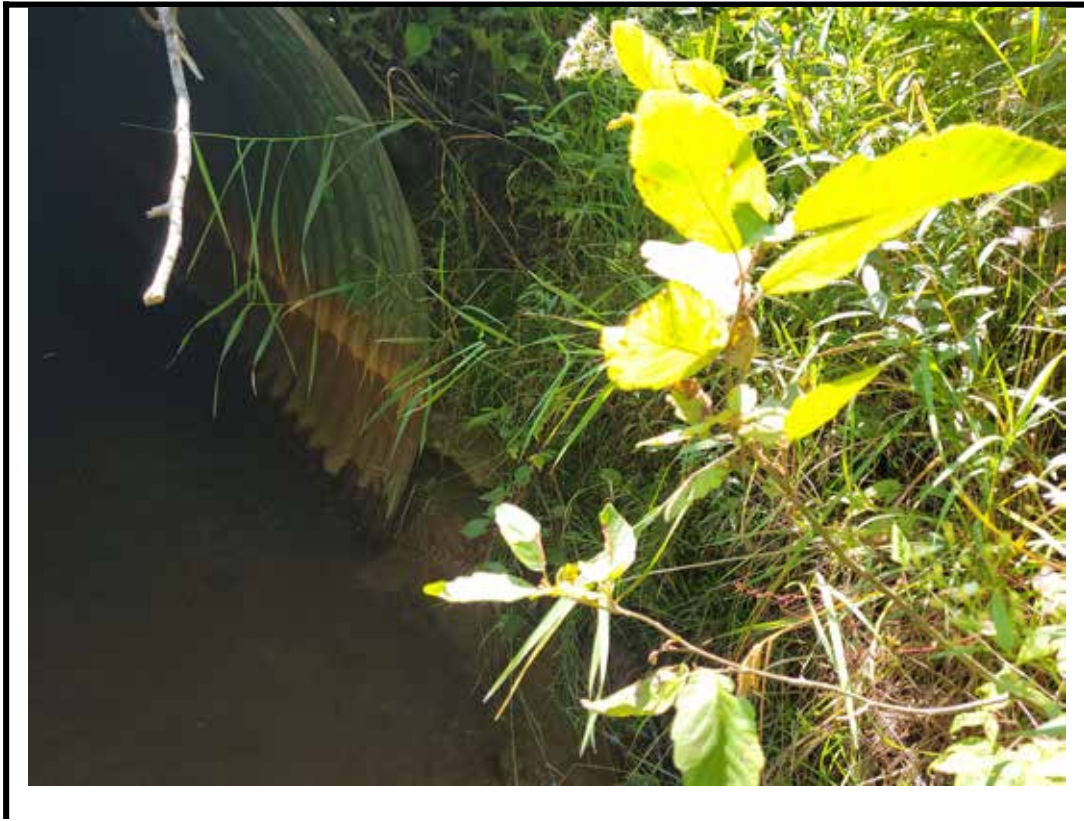
Photo 9 Moderate erosion of embankment at north end of barrel
