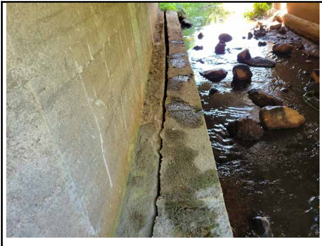
Photo 12 Separation of concrete footing at south abutment wall
