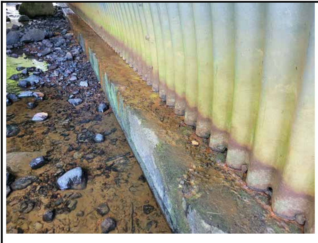
Photo 8 Small spalls and light to moderate scaling on exposed concrete footing
