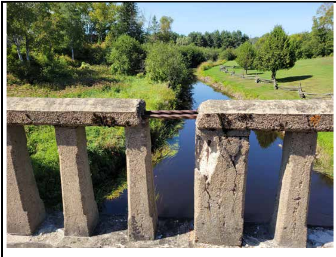
Photo 8 Large section loss of concrete railing
