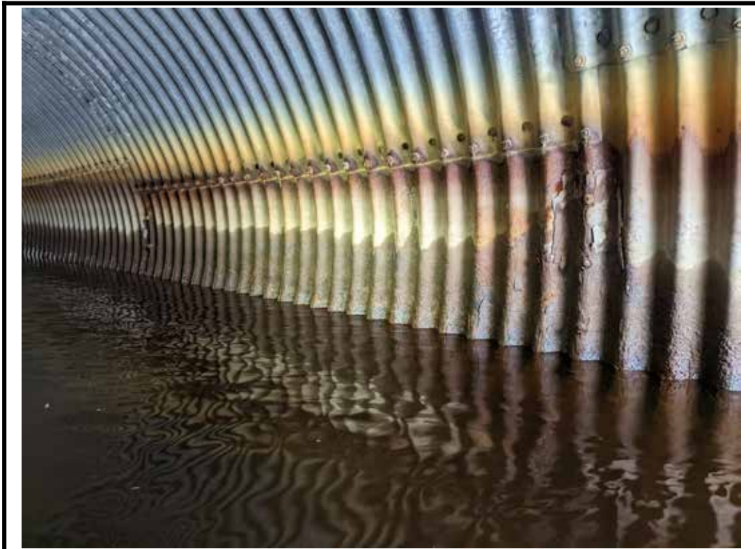
Photo 9 Corrosion at high water level
