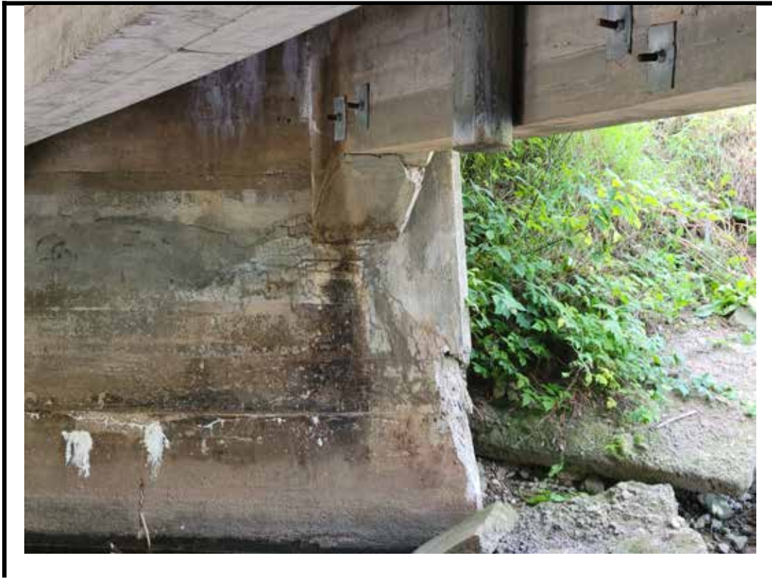
Photo 15 Narrow to medium cracks with damp stains and efflorescence on north abutment
