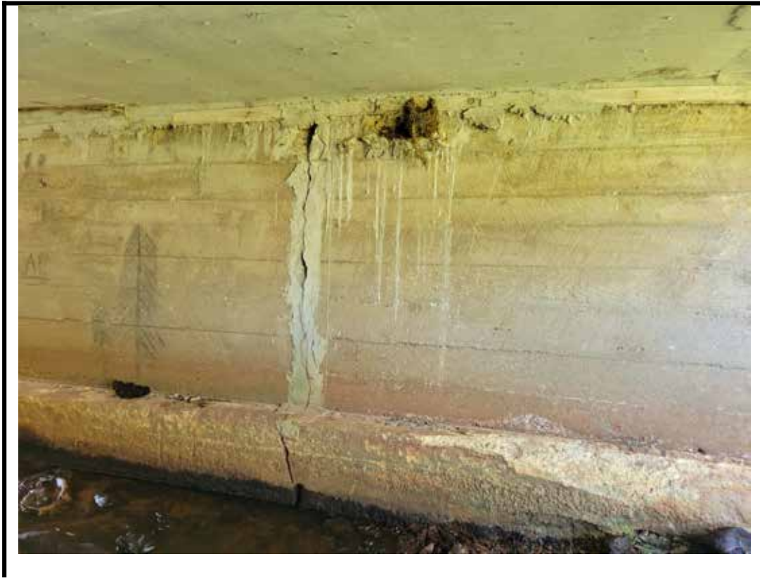
Photo 13 Severe scaling and disintegration at base of north abutment wall
