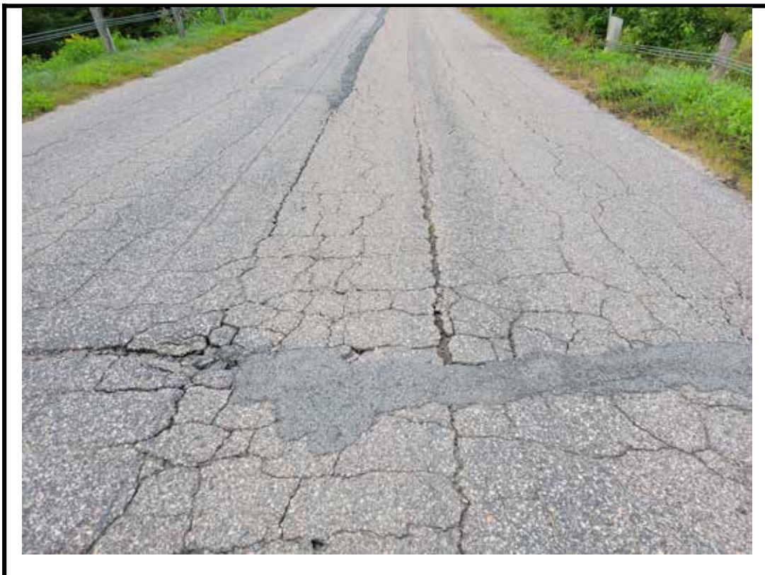
Photo 10 Patched potholes and wide map cracking on south approach wearing surface
