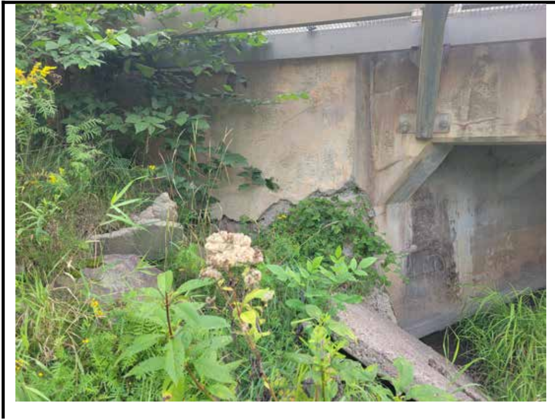
Photo 11 Isolated severe disintegration on SE wingwall
