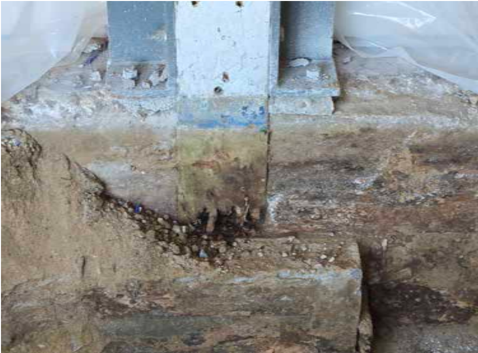
Photograph 1: Deterioration below slab - interior column
