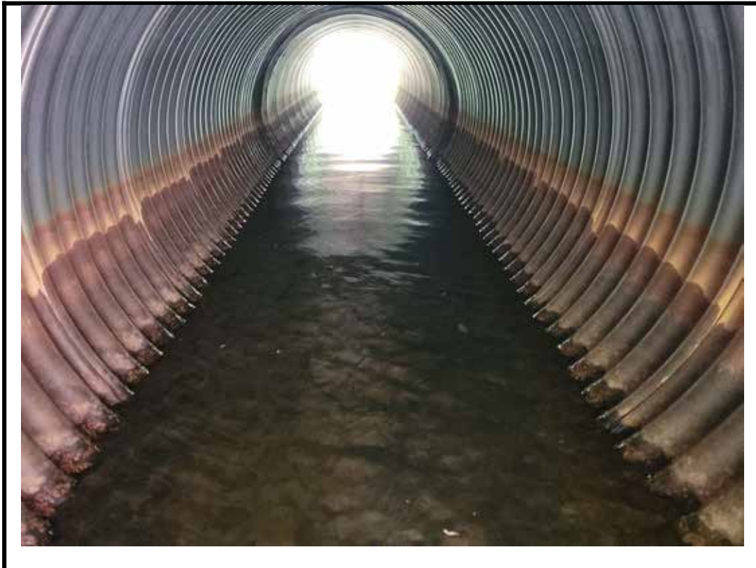
Photo 8 Light corrosion observed along waterline
