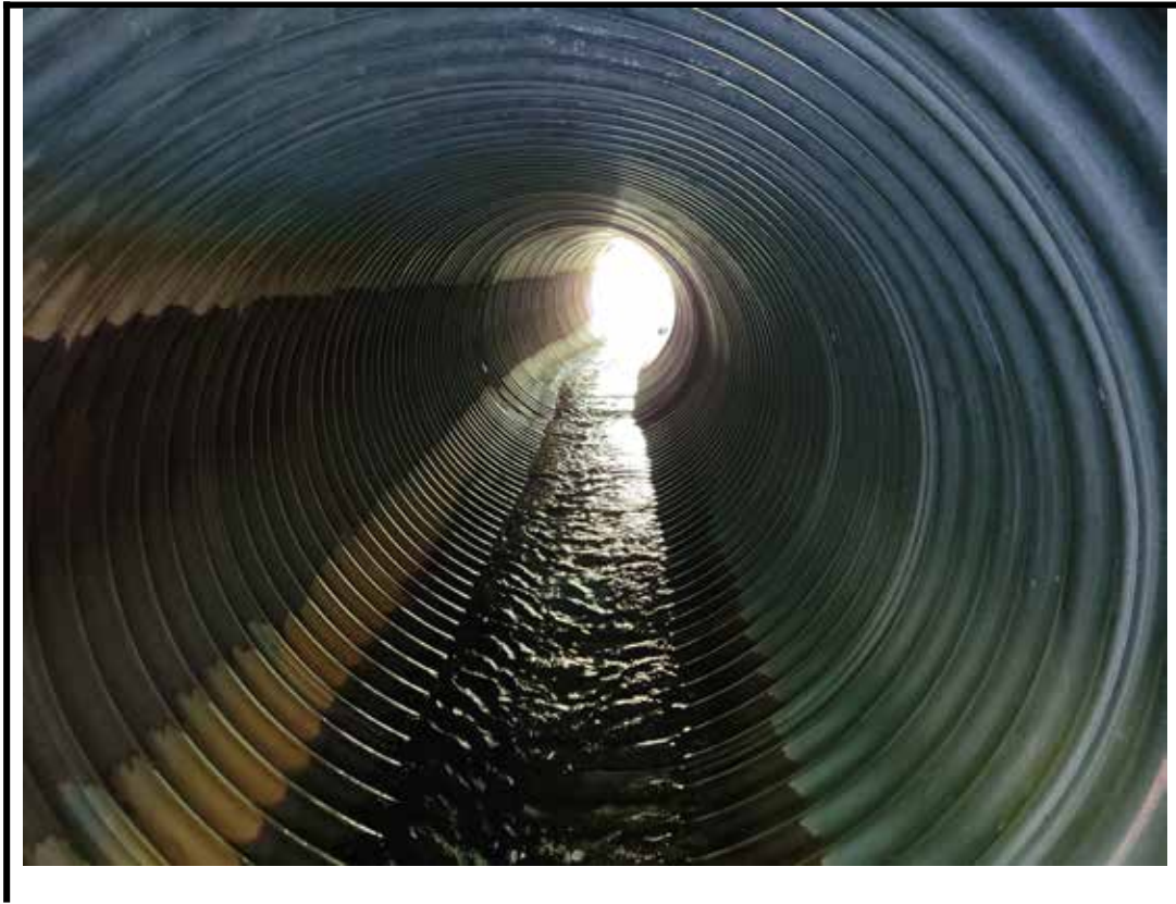
Photo 7 Light corrosion at and above high water level
