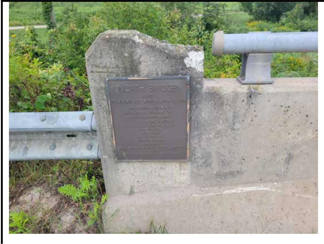
Photo 7 Substandard guiderail structure connection and spall at end of parapet wall
