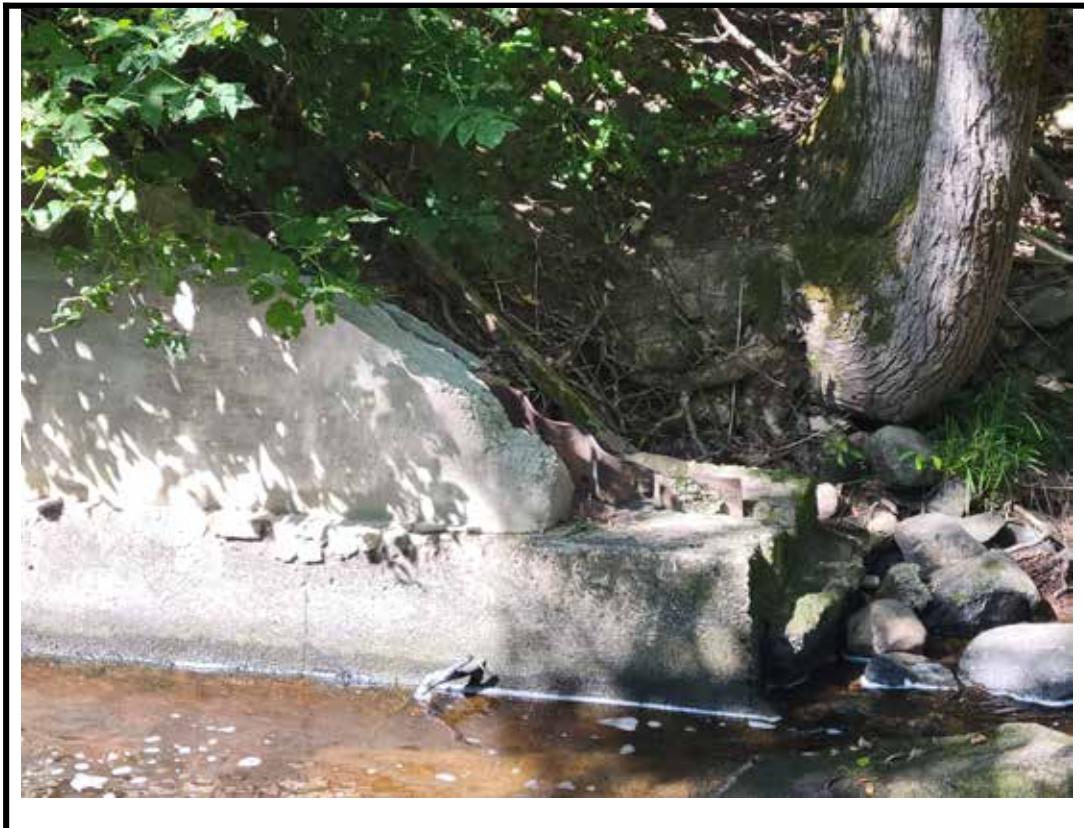
Photo 12 Localized light honeycombing on concrete repair at north end of structure
