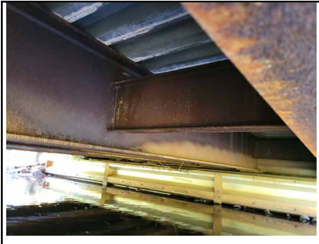
Photo 10 Localized light corrosion on steel girders and diaphragms
