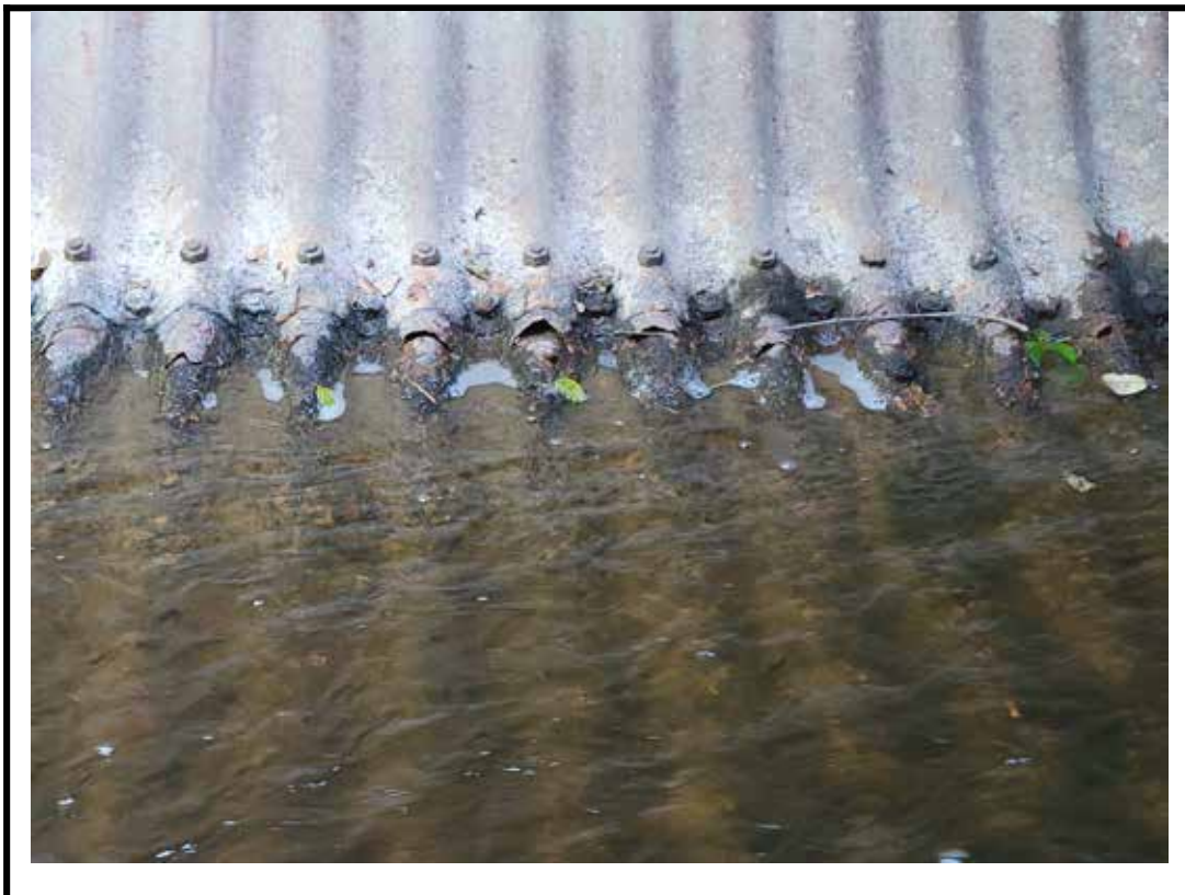
Photo 12 Localized severe corrosion with perforations on bottom of barrel (east end shown)
