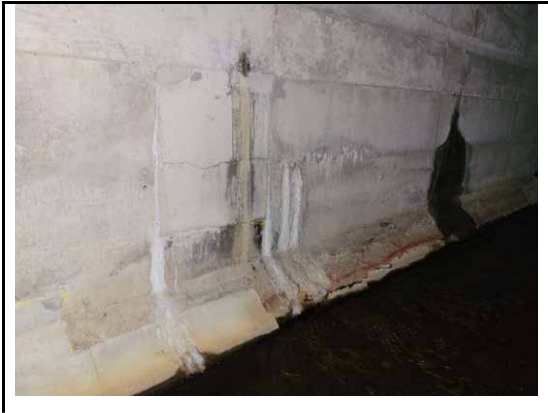
Photo 11 Narrow to medium horizontal crack with efflorescence on south wall of barrel
