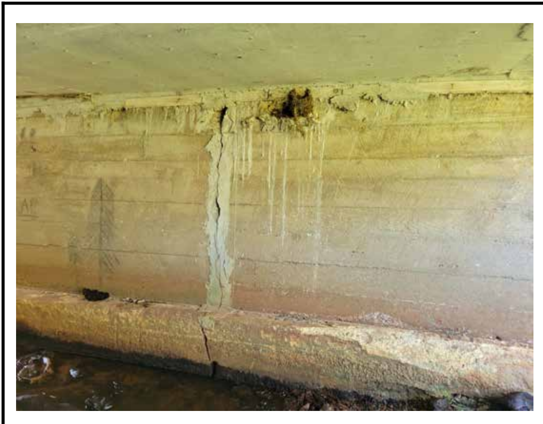
Photo 10 Vertical crack on north abutment wall
