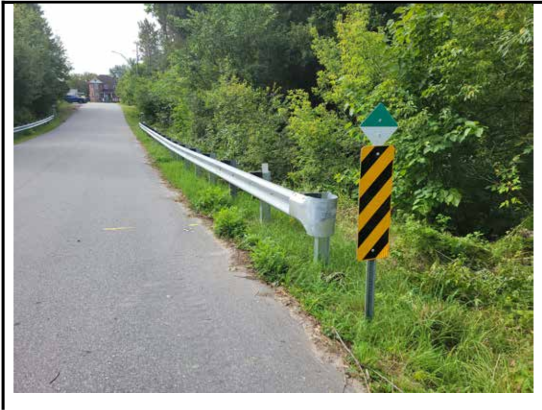
Photo 7 Substandard guide rail end treatment at NW approach guide rail
