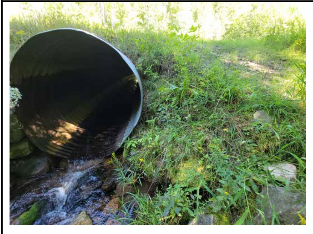
Photo 10 Erosion of embankment at east end of barrel
