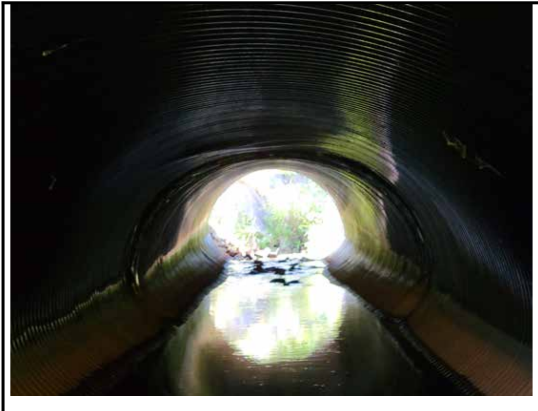
Photo 8 Deformation of culvert under roadway
