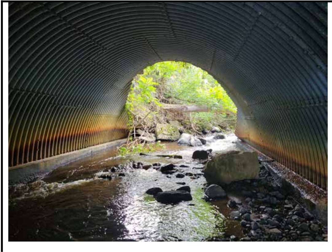
Photo 11 Accumulation of rocks in east end of barrel
