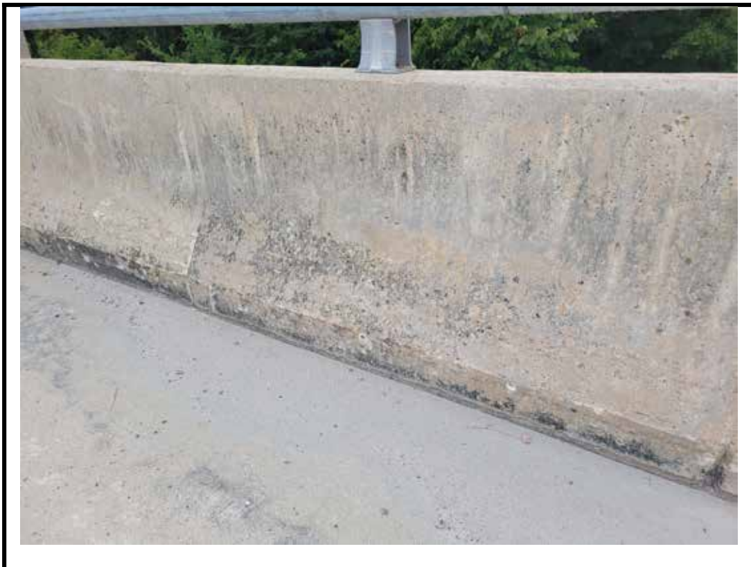
Photo 10 Narrow cracks and scaling noted on parapet wall
