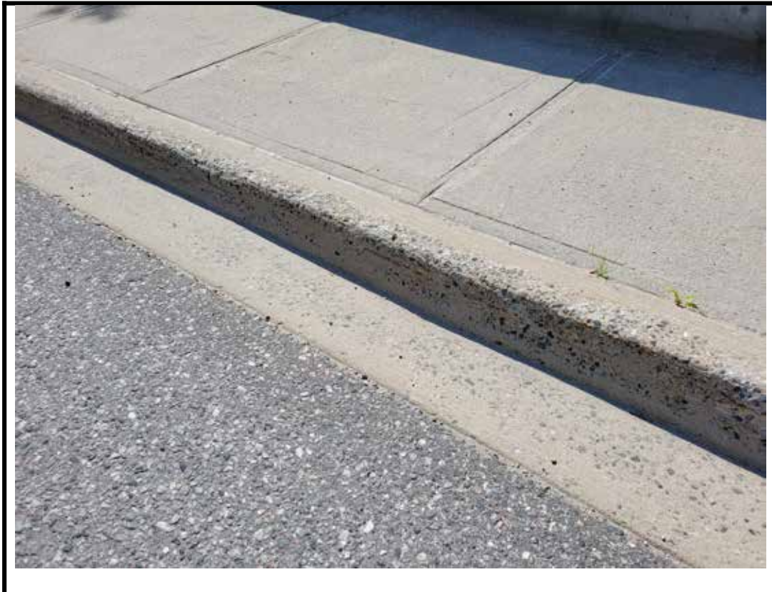
Photo 9 Abrasions and light to moderate scaling on concrete curb
