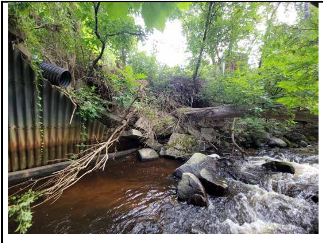
Photo 12 Accumulation of branches and debris on NE embankment
