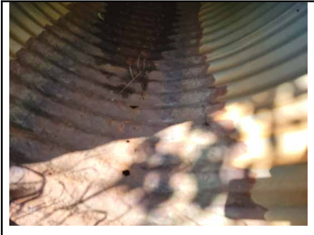
Photo 9 Localized severe corrosion with perforations in bottom of barrel
