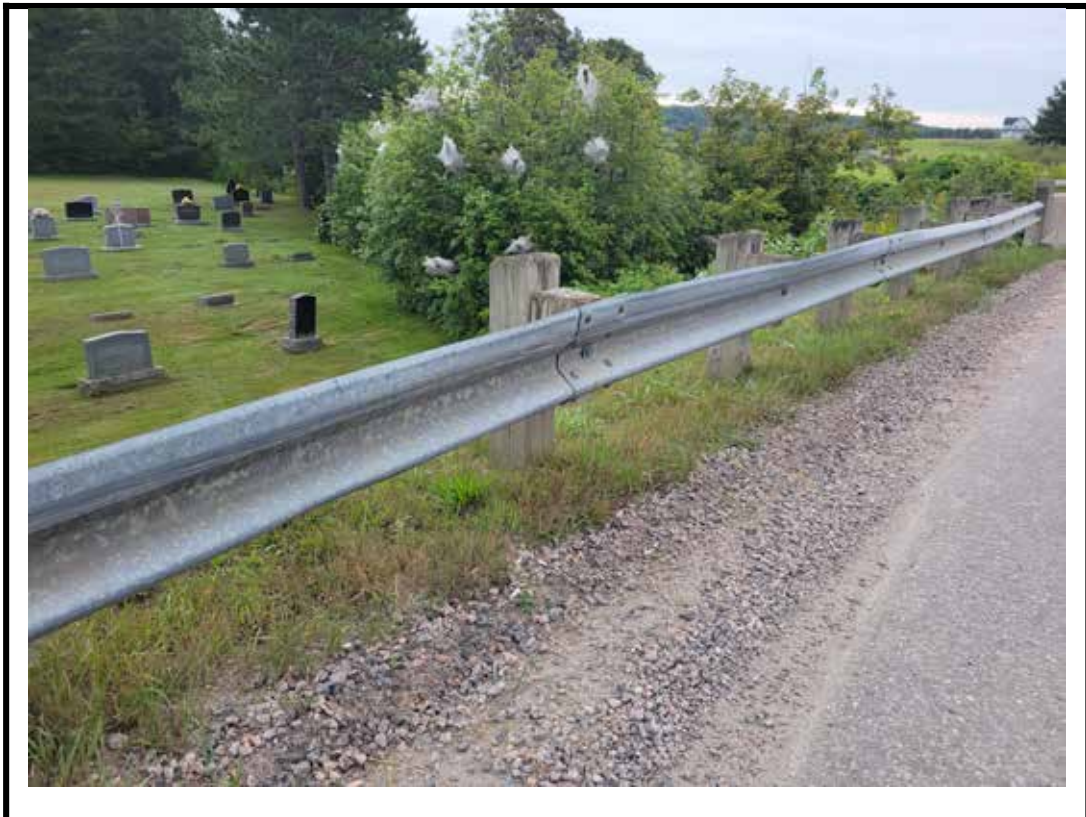
Photo 8 Deformation and abrasions on NE approach guide rail
