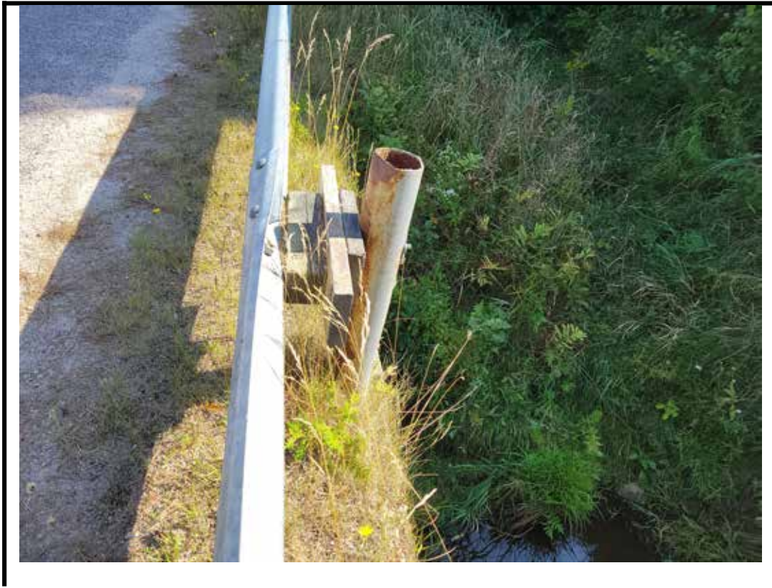
Photo 9 Circular HSS with timber blocking on west barrier
