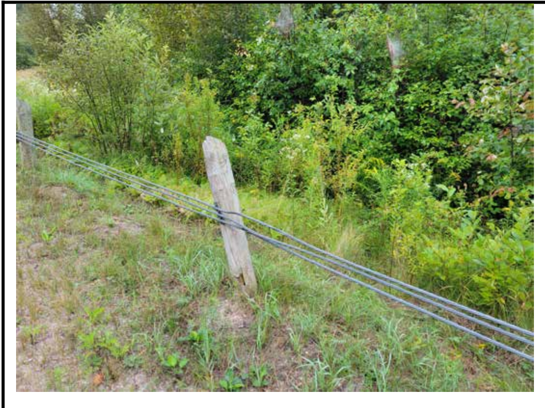
Photo 7 3 Cable guide rail with loose cables on approaches
