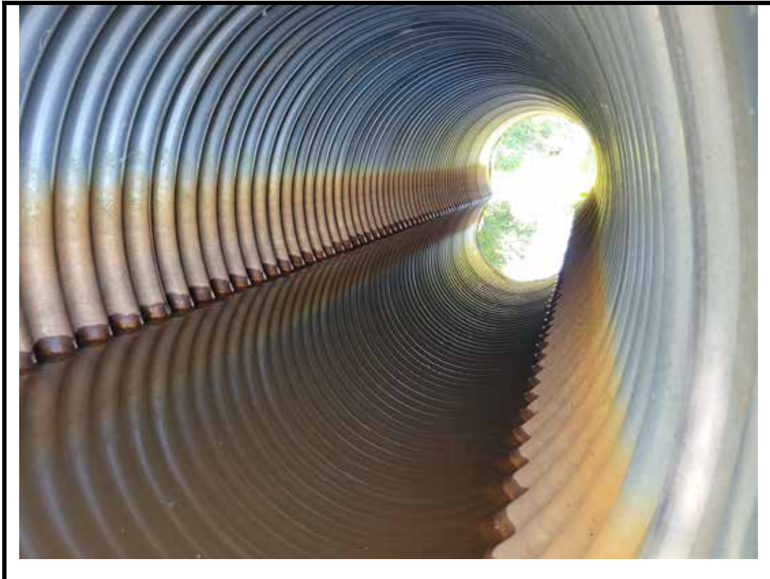
Photo 8 Light corrosion noted at waterline
