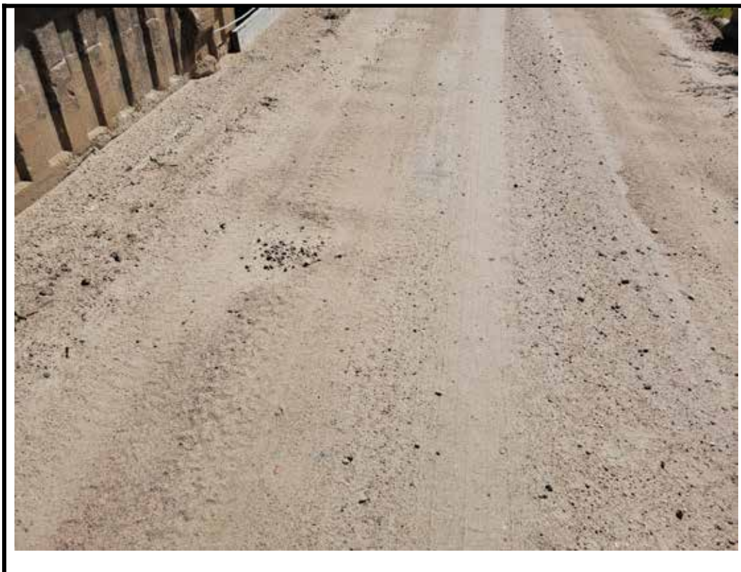
Photo 11 Potholes and wheel rutting noted on asphalt wearing surface
