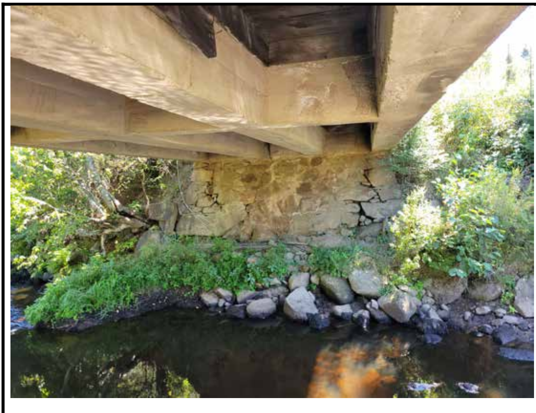
Photo 12 Deck drain downspout does not extend below girders
