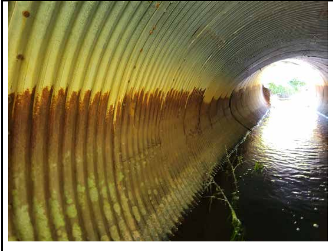
Photo 10 Moderate corrosion below the high water line throughout barrel
