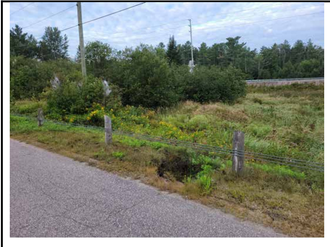
Photo 9 Localized severe erosion of shoulder on the west side of the roadway
