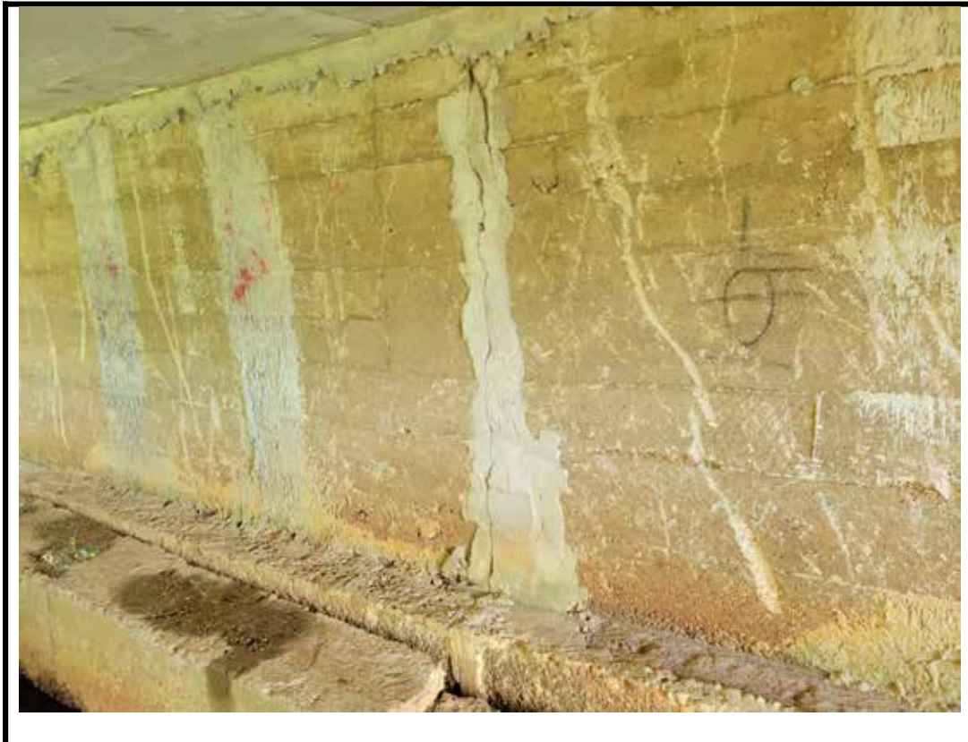
Photo 11 Vertical crack on south abutment wall at mid-section
