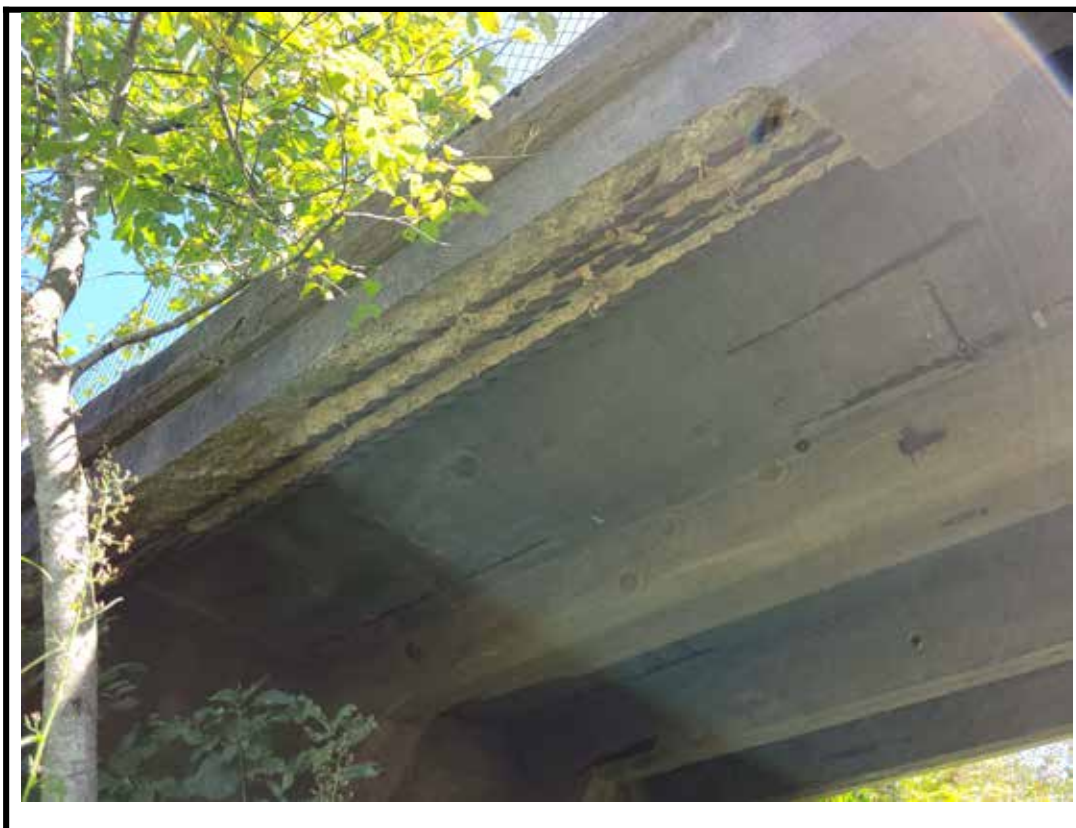
Photo 10 Spalls with exposed corroded reinforcing on exterior girder and interior soffit
