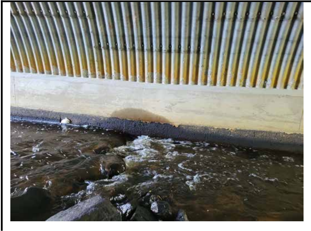
Photo 13 Isolated damp staining between concrete repair and existing exposed footing on west side of barrel
