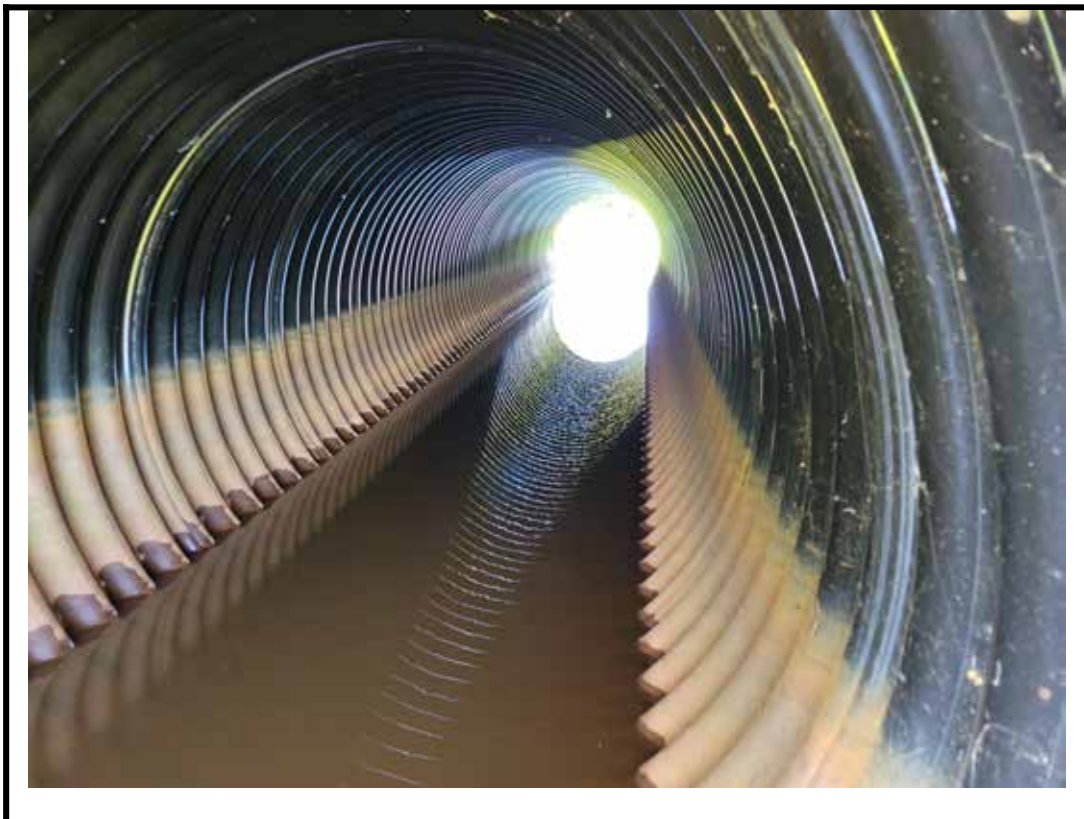
Photo 8 Light corrosion below the high water line throughout the barrel
