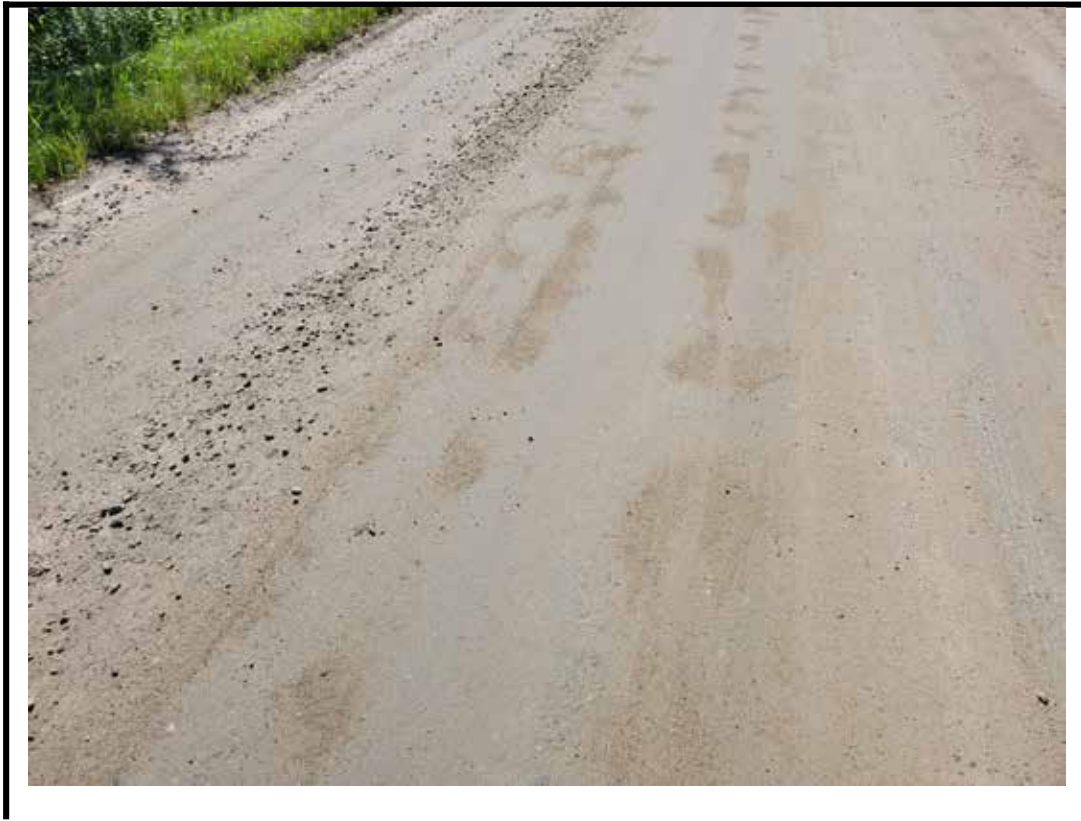
Photo 7 Small spalls on approach wearing surface
