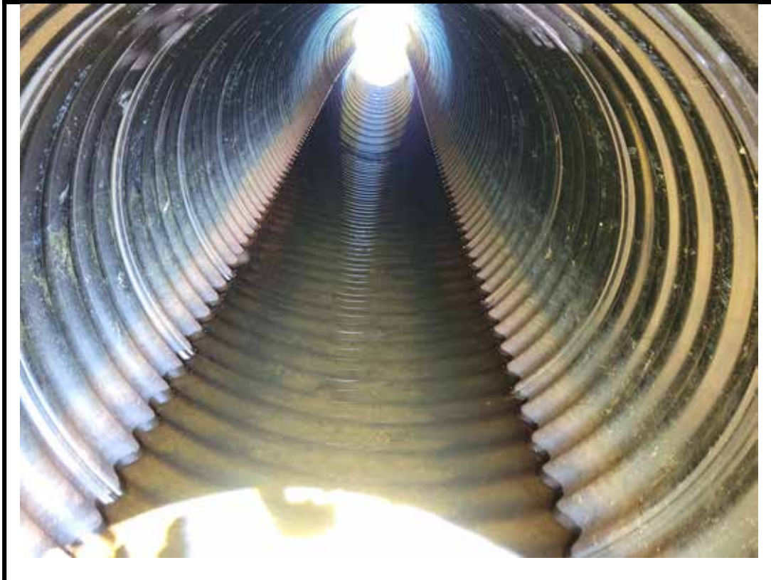
Photo 8 Light weathering of interior of barrel
