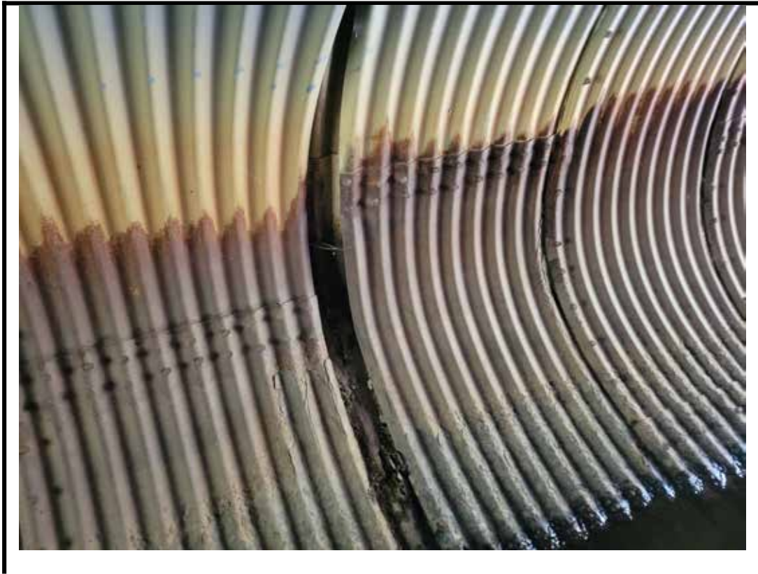
Photo 11 Separation of barrel
