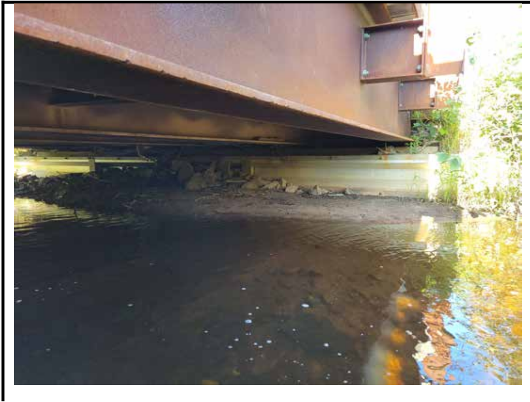
Photo 13 Sediment accumulation at east abutment wall
