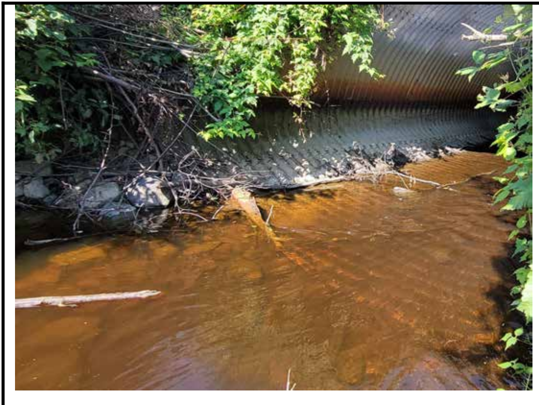
Photo 12 Deformation of bottom of the south end of the barrel
