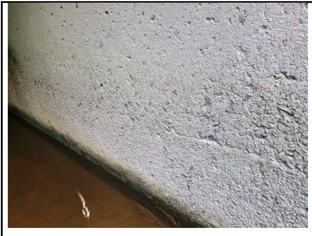
Photo 12 Localized light to moderate scaling on north barrel wall
